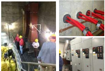
Site visits conducted to assess vulnerable facilities & identify practical, cost-effective measures to mitigate climate threats.
