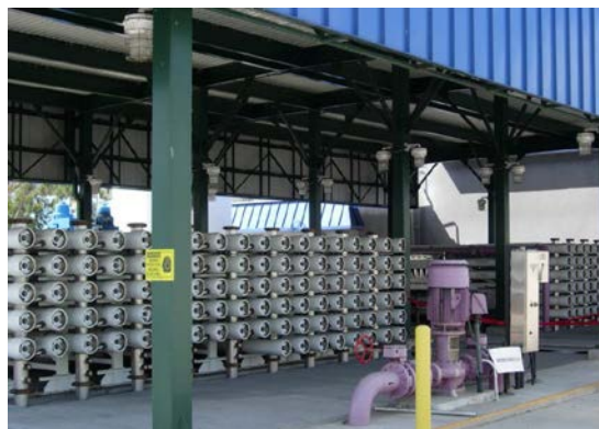
The advanced treatment capacity at TIWRP was recently expanded to 12 mgd enabling TIWRP to recycle 100 percent of its wastewater with advanced water purification.
