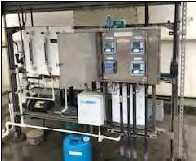
Finished Product Water Quality instrument cabinet
