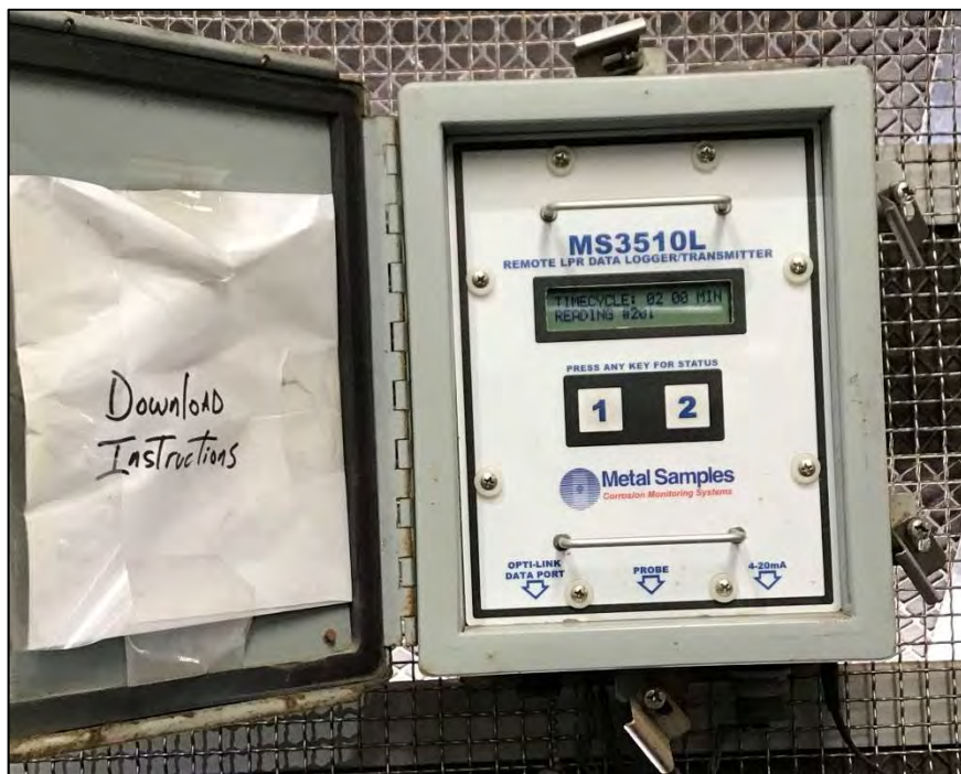
Close up image of LPR download interface unit (Hoffman Box).
