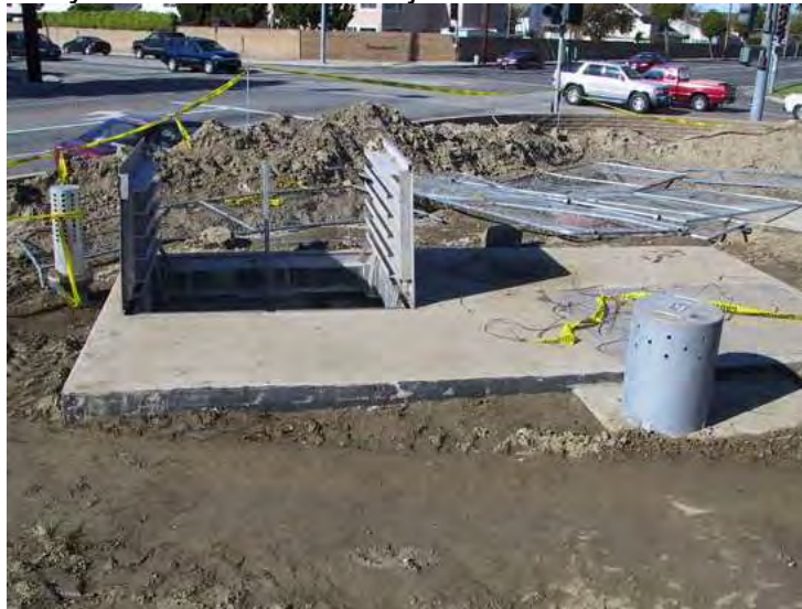
View of PRV-2 vault looking north to Ellis and Ward intersection
