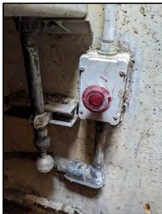
Figure 23 Near the bottom of the vault access ladder is an e-call button that sends a distress alarm to Delta V. Also in view is the secondary flood alarm float switch. This stainless steel ball is very sensitive and will automatically cut-off all injection into that Legacy Well if activated. (Not something the IRSO wants to accidentally bump into.)
