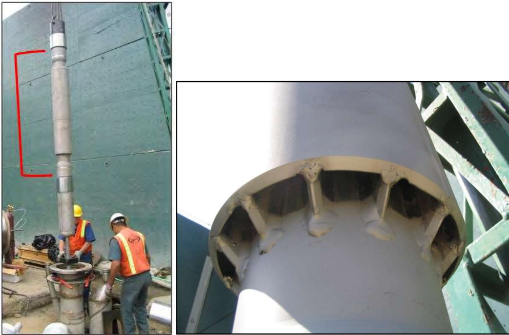
Figure 36 Baski Valve identified by the red bracket in the left image. A close up of the valve discharge port is shown in the right image. Note the 2-inch dedicated airline passing through the Baski Valve and bullnose pipe end-piece at the end of the assembly. This allows greater airline submergence for shallow Modern Well settings.
