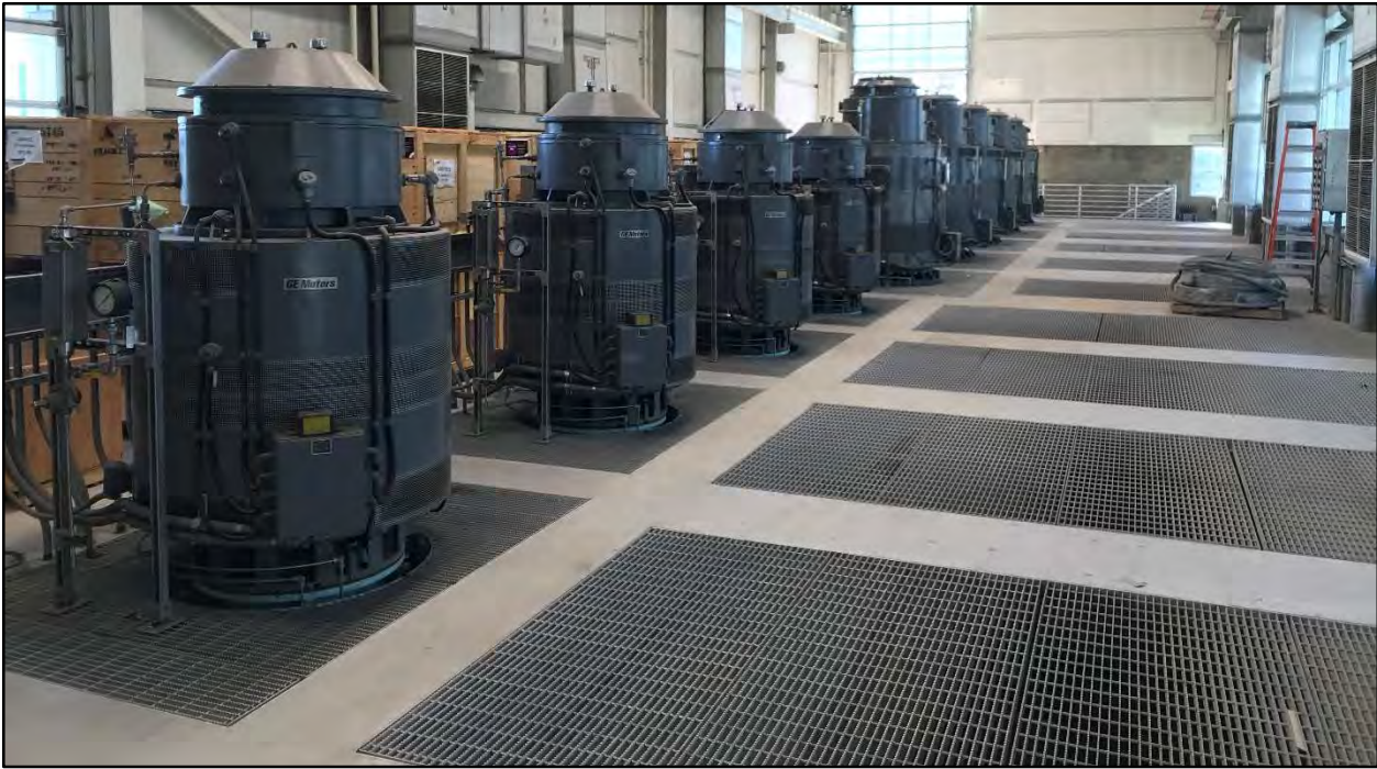
Figure 47 GWRS Final Product Water Pump Station. The four shorter pump motors in the foreground power the Barrier Product Water Pumps. The larger motors in the background power the pumps that lift GWRS water over 200 feet in elevation to the recharge spreading grounds in Anaheim.
