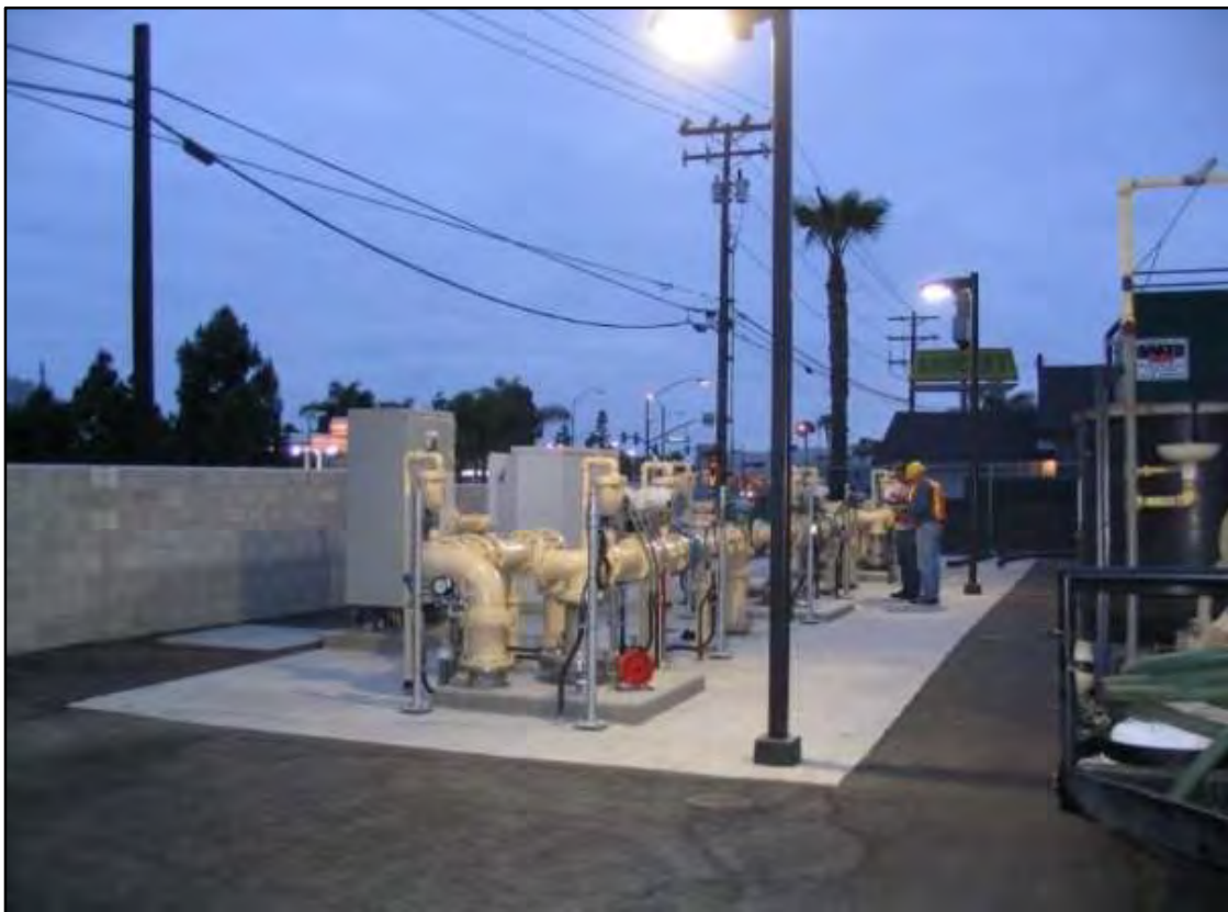
Modern Injection Well Site I-32.
