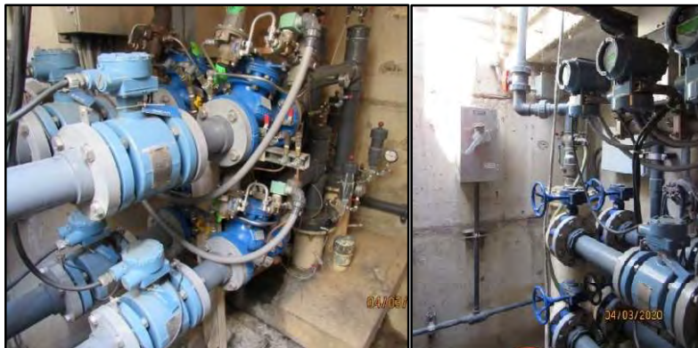
Figure 19 Views looking inside a typical Legacy Well vault. Legacy Well vaults are compact requiring the IRSO to be aware of their surroundings. The Legacy Well well-head is visible in the left image. The Legacy Well components visible in these images are defined later in this manual.
