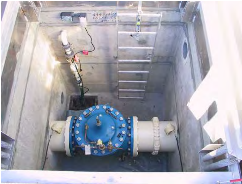
View into PRV-1 vault. Sump pump can be operated with portable generator.
