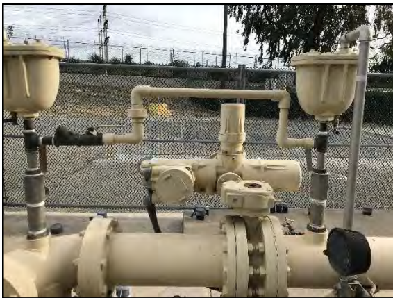
Figure 37 1-inch MOV bypass line. These lines are installed at: I-24, I-25, I-26, I-27 and I-28 and used to combat eductor pipe leakage from the couplings when the Baski Valve is closed.
