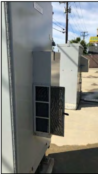
Figure 40 Modern Well Process Control Cabinet. Note the air conditioner unit mounted to the door. The air conditioner filter removes by gently pulling on the tab down. The filter in this image is partially removed. The IRSO removes, rinses and reinstalls these filters monthly as a preventative maintenance activity.
