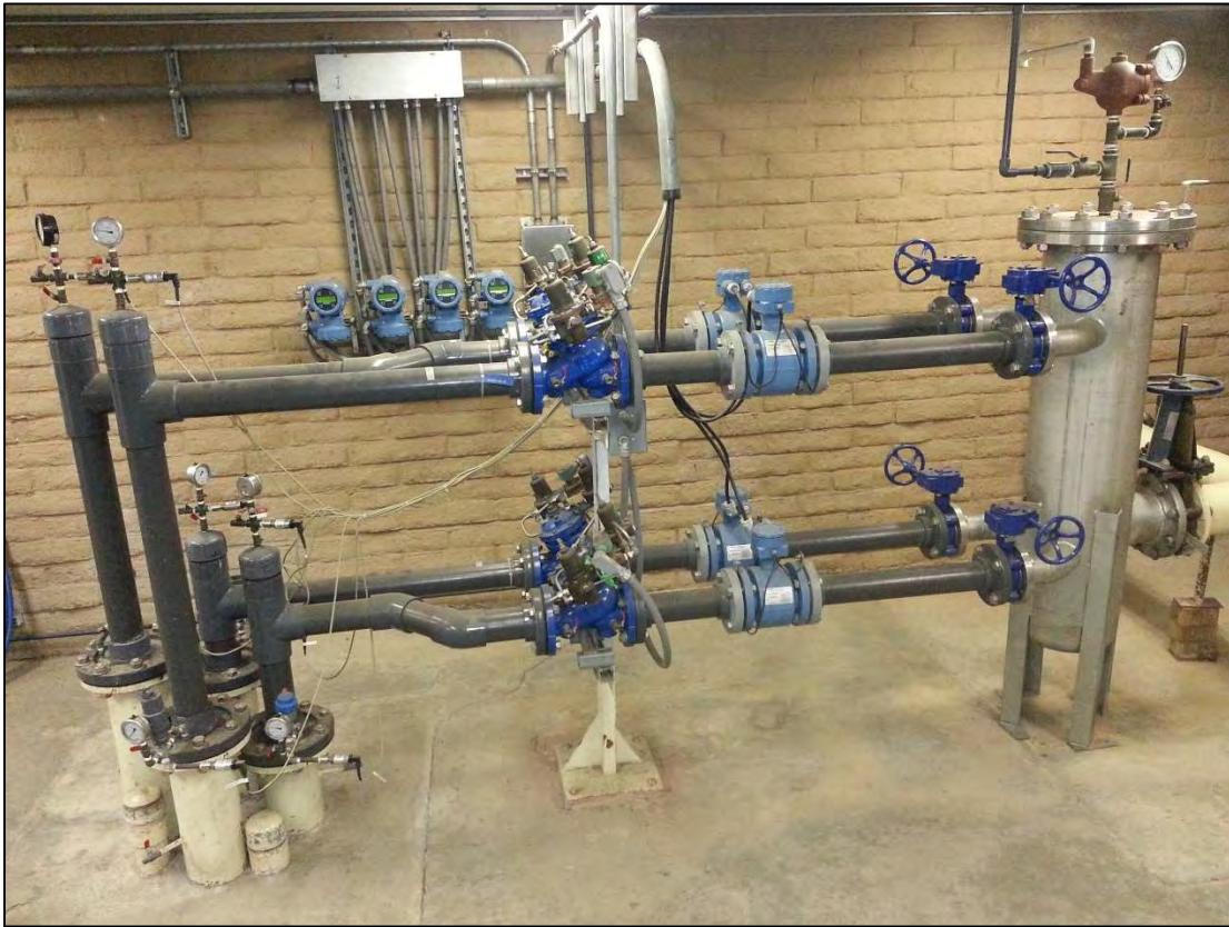
Figure 5 Legacy Well I-4. I-4 contains four 6-inch casings targeting the Talbert, Alpha, Beta and Lambda aquifers. Legacy Well I-4 is the only Legacy Well completed above ground surface.
