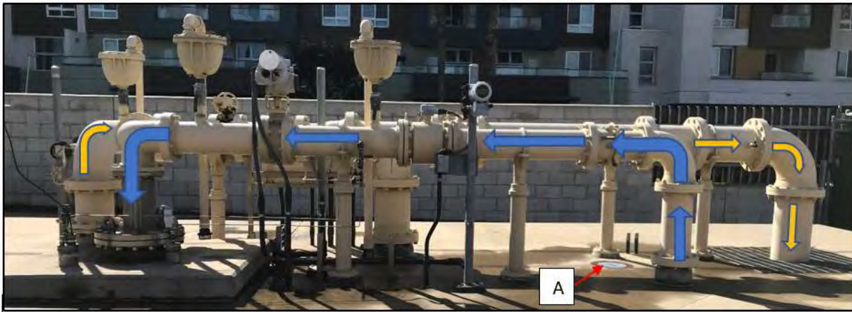
Figure 32 Typical Talbert Seawater Intrusion Barrier Modern Injection Well. Blue arrows indicate the flow path from the lateral pipeline into the well casing. Orange arrows indicate the backwash discharge flow direction. A Lateral isolation butterfly valve operator.
