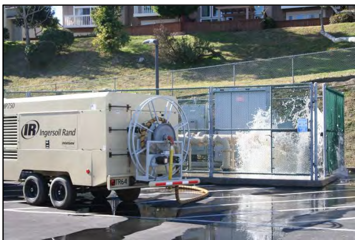
Figure 37 Airlift backwashing Modern Well I-29 utilizing the District-owned portable air compressor (TR-64). This image was captured the moment when air-lift break over pressure was achieved and discharge first reached atmosphere. Most of the time discharge is fully contained within the on-site storm drain catchment basin.
