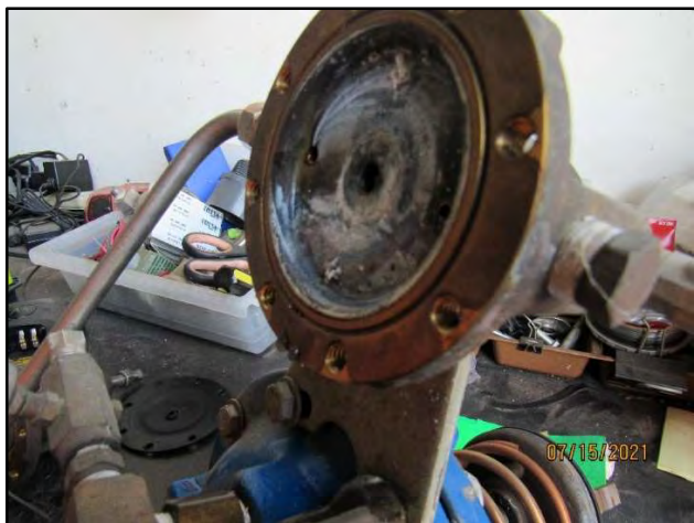
Figure 27 PRV valve diaphragm being prepared for replacement . A new replacement diaphragm is visible in the lower left quadrant of this image.
