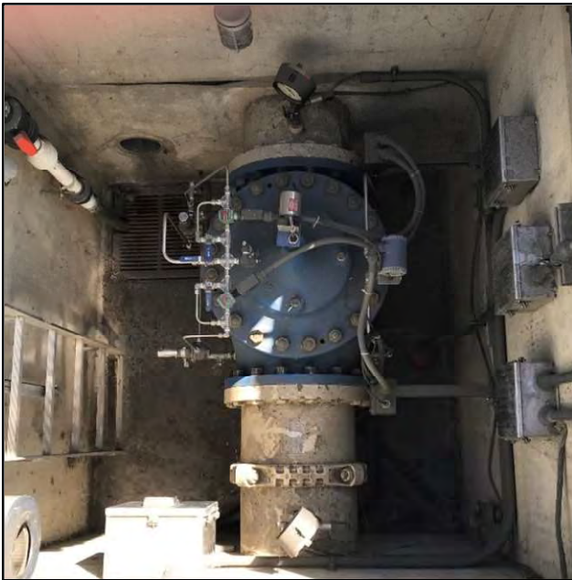
Figure 13(B) Inside the vault showing the OC-44 flow control valve.
