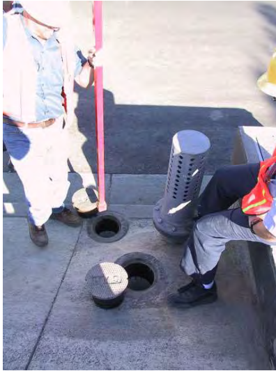
Typical valve can installation. All valve lids are marked with GWRS.
