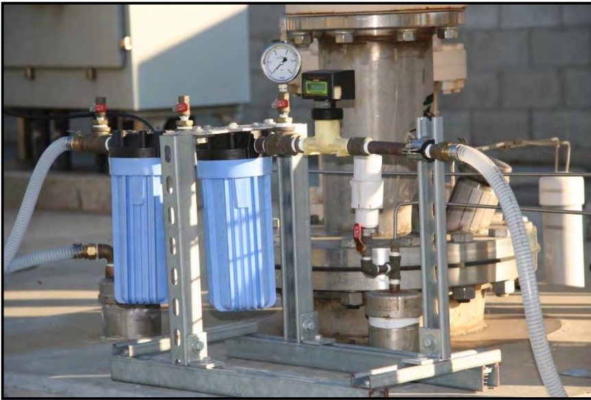
Figure 15 (A) 5 and 1 micron bypass filter test skid used to determine the amount of solids being delivered into the injection wells. There are several of these skids located throughout the Talbert Barrier distribution system.
