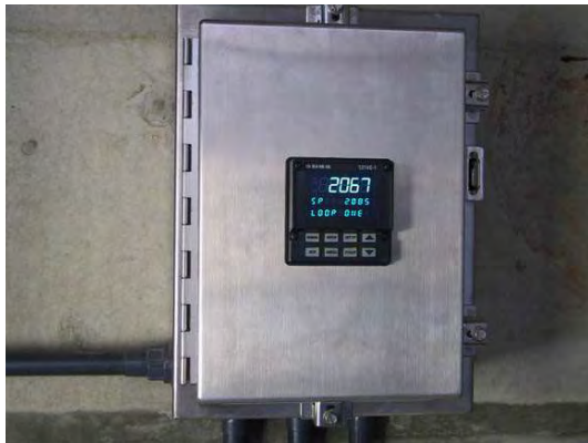
Downstream Flow Control Box
