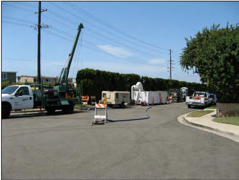
Figure 29 Injection Well redevelopment contractor working on Legacy Well I-14 (Ellis @ Bushard). The contractor is air-lift pumping the well to dislodge and remove fine grained particles that accumulate in the well screen and adversely impact well performance. Air-lift pump discharge is desilted in the white baffled tank and placed in the local sewer. The discharge will be return to GWRS for treatment and future injection.
