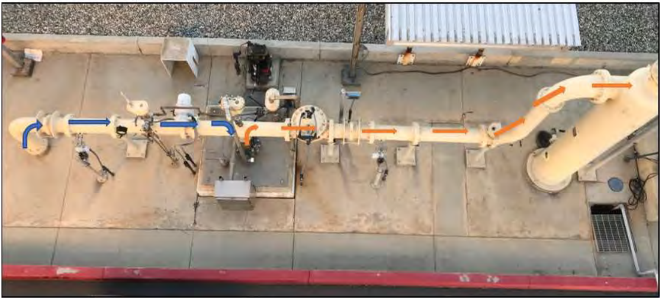
Figure 42 Hybrid Well I-25. Blue arrows indicate the flow path from the exposed lateral pipeline into the injection well. Orange arrows indicate the backwash discharge flow path to waste.
