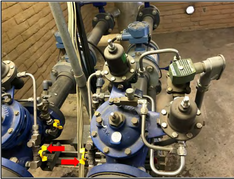
Figure 46 Legacy Well pressure reducing valve (PRV). Red arrows indicate the location of “Cock 2”. The IRSO can secure flow to a PRV that is nonresponsive to Delta V by manually closing cock 2 or by closing the upstream butterfly valve. When pipeline pressure is restored Cock 2 will automatically reset and be ready for a remote restart. If the IRSO chooses to secure flow with the butterfly valve, a second well site visit is required upon start-up to open the butterfly valve.
