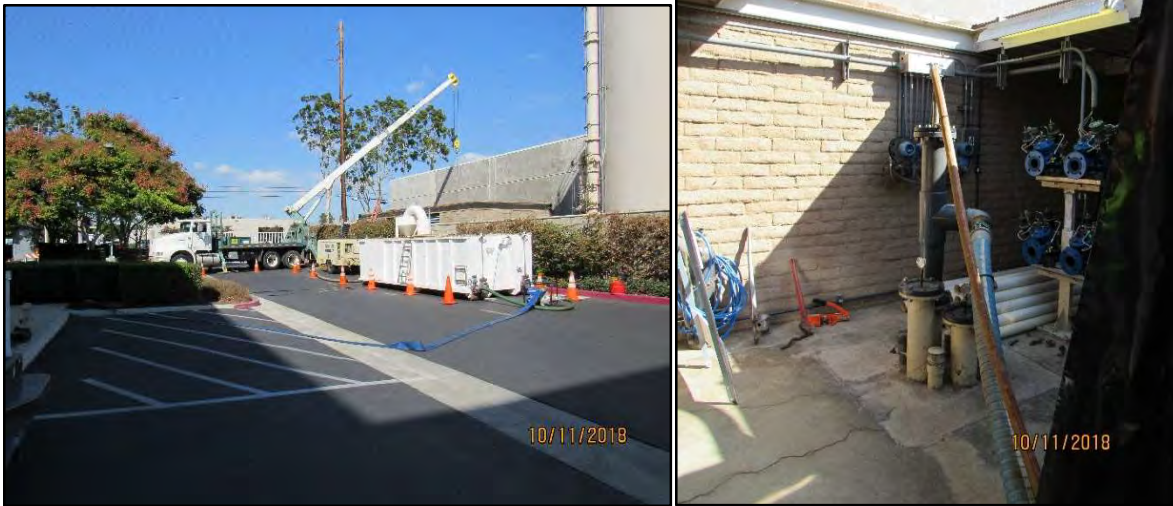
Figure 17 Demonstration building that houses the I-4 well-head, located in the northeast corner of the Fountain Valley campus. Removable metal roof panels allow access for well
