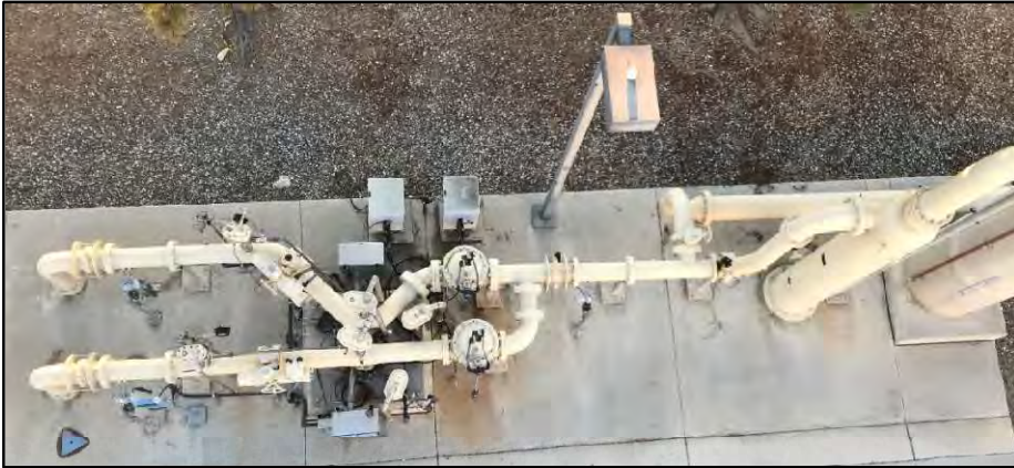
Figure 41 Hybrid Well site I-24 (above) and I-25 (below) located on the OCWD Fountain Valley campus along the East Perimeter Road. I-24 is nested with 2 casings in 1 bore hole. I-25 is a single casing well. Although these two wells are only separated by 420 feet, the geology is different, hence, the different well completions. Geologists claim that a splay of the Newport Inglewood Fault Zone runs between the two Hybrid wells.
