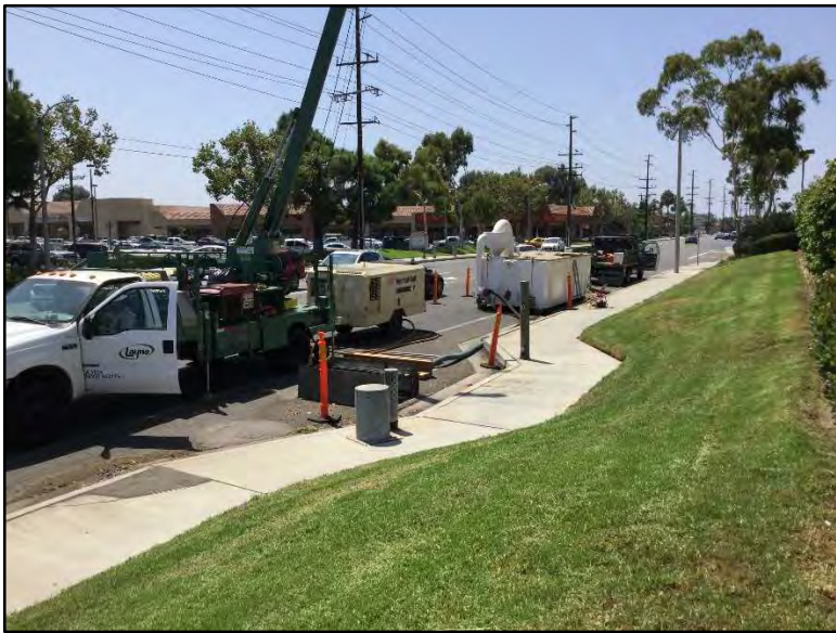
Figure 20 Most Legacy Wells are located in public right-of-way. Legacy well I-10, shown here, is located at the NE corner of the intersection of Ellis Avenue and Brookhurst Street. Notice the vault manway hatch double leaf doors are open. The well-head access hatch has been removed and boards are covering the opening. The white portable desilting tank is owned by OCWD to aid in maintaining backwash discharge compliance.
