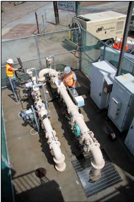
Figure 38 Two IRSO's backwashing Modern Well I-36. The operator on the left is controlling the air from the compressor into the well. The operator on the right is monitoring and documenting the discharge water quality for regulatory compliance. The well can be seen discharging into the storm drain catchment basin.
