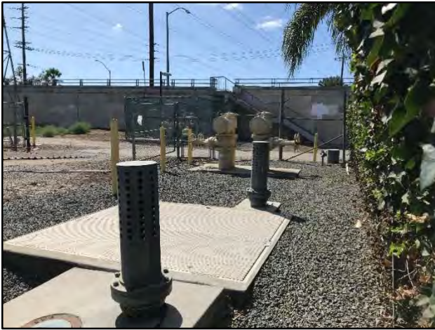
Figure 13(A) Image looking south showing the OC-44 flow control valve vault. The backflow prevention device is behind the vault. Modern Injection Well I-36 can barely be seen behind the backflow device.
