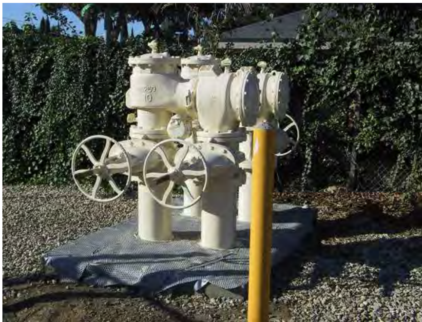
Backflow device located north of Adams Frontage Road. Devices are required to be tested and certified annually.
