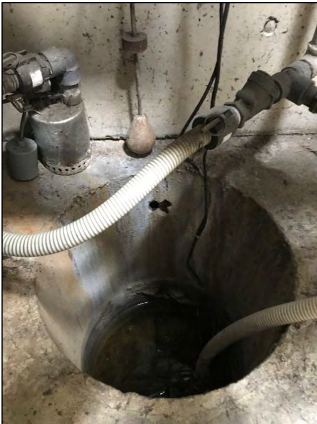
Figure 24 A typical Legacy Well vault sump. The supporting sump pump and float switch is visible on vault floor. The lead pump discharge tubing is seen leaving the sump and cam lock connecting to the PVC discharge line. Also present is the lowest (floor elevation) vault flood alarm float switch (just to the right of the supporting sump pump). The perched groundwater weep hole cored high into the sump wall can be seen at 12:00 o'clock.
