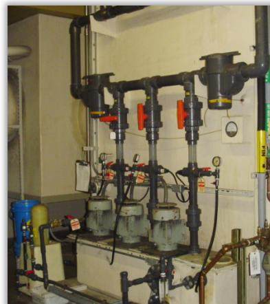
Figure 7.17 - Fume Scrubber for a Microelectronics Lab
