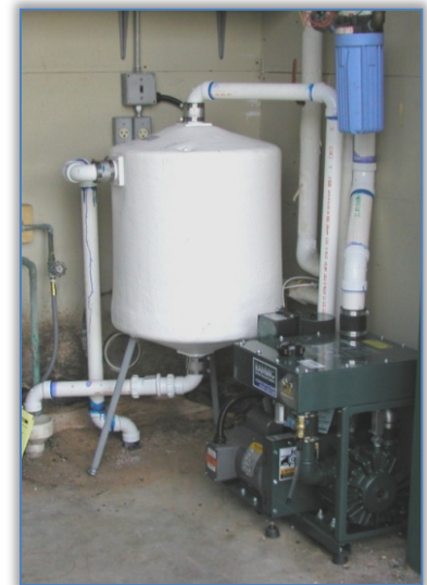
Figure 7.15 - A Dry Vacuum System at a Dental Office
