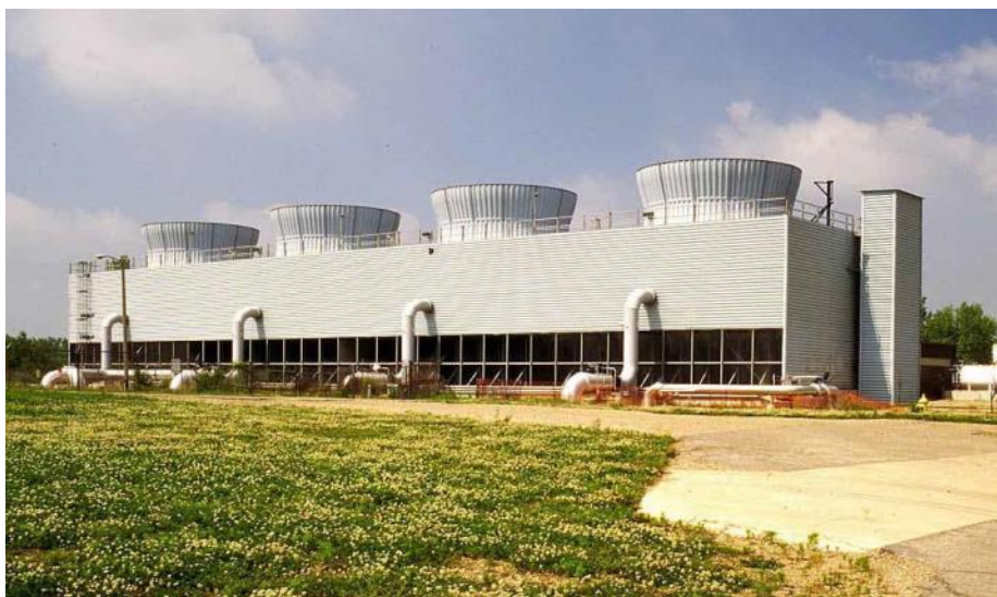
Figure 7.50 - Marley Counter-Flow Towers
