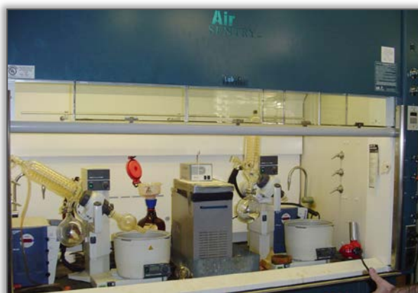
Figure 7.16 - A Typical Hood System in a Lab
