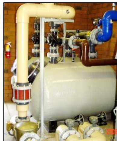
Figure 7.63 - Large Sand Filters of a Public Pool
