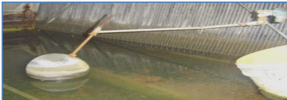
Figure 7.51 - Cooling Tower Float Valve and Overflow Pipe
