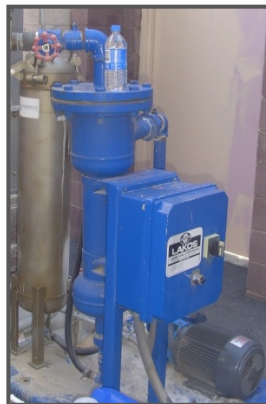
Figure 7.68 - Cyclone Separator with Bag Filter
