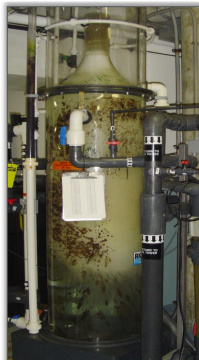
Figure 7.22 - Large Aquarium Sand Filters
