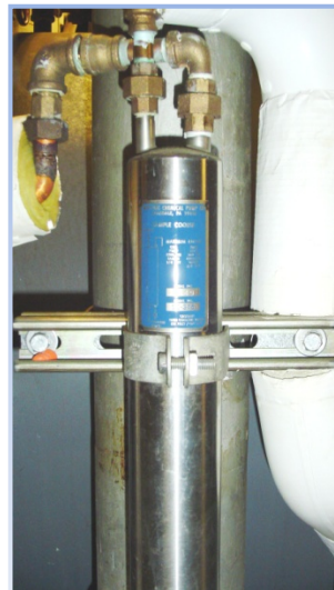
Figure 7.57 - Boiler Water Sampler Device
