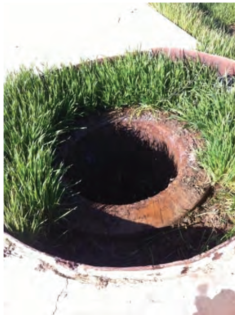
Figure 2-2. Existing Wellhead with Cover Removed
