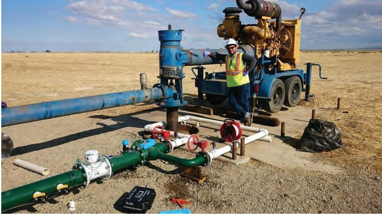
Figure 2-12. Wellhead Control and Other Equipment
