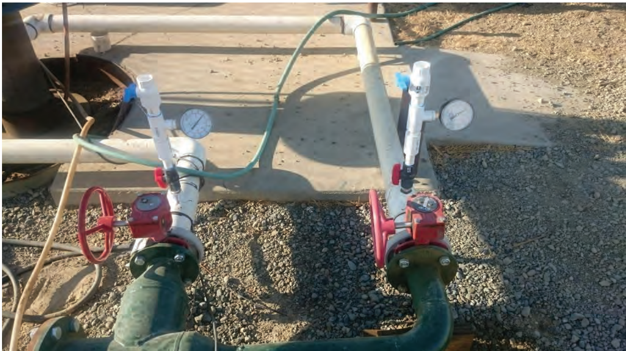
Figure 2-13. Injection Control and Air Bleed Valves with Added Combination Pressure/Vacuum Gauges
