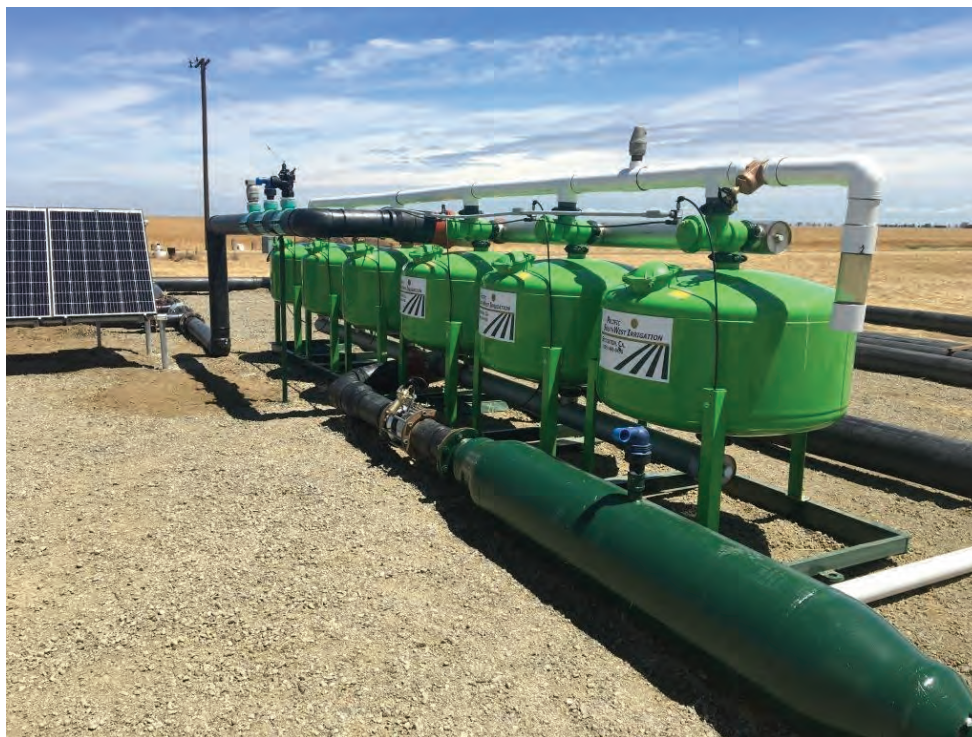
Figure 2-11. Filters and Air Release Chamber
