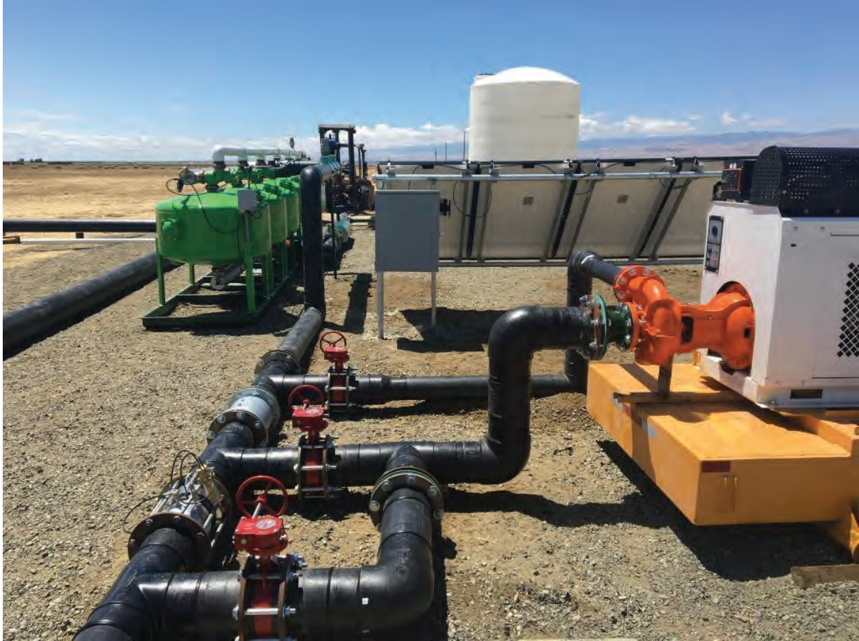
Figure 2-10. Booster Pump and Upstream Valves at Initial Installation
