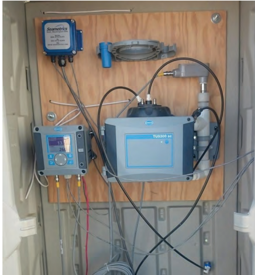
Figure 2-16. Instruments Inside Instrument Shed
