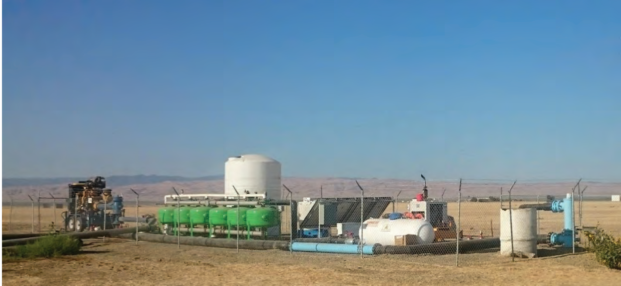
Figure 2-9. Installed Equipment and Related Facilities
