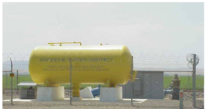
Panoche Drainage District Recirculation Plant
