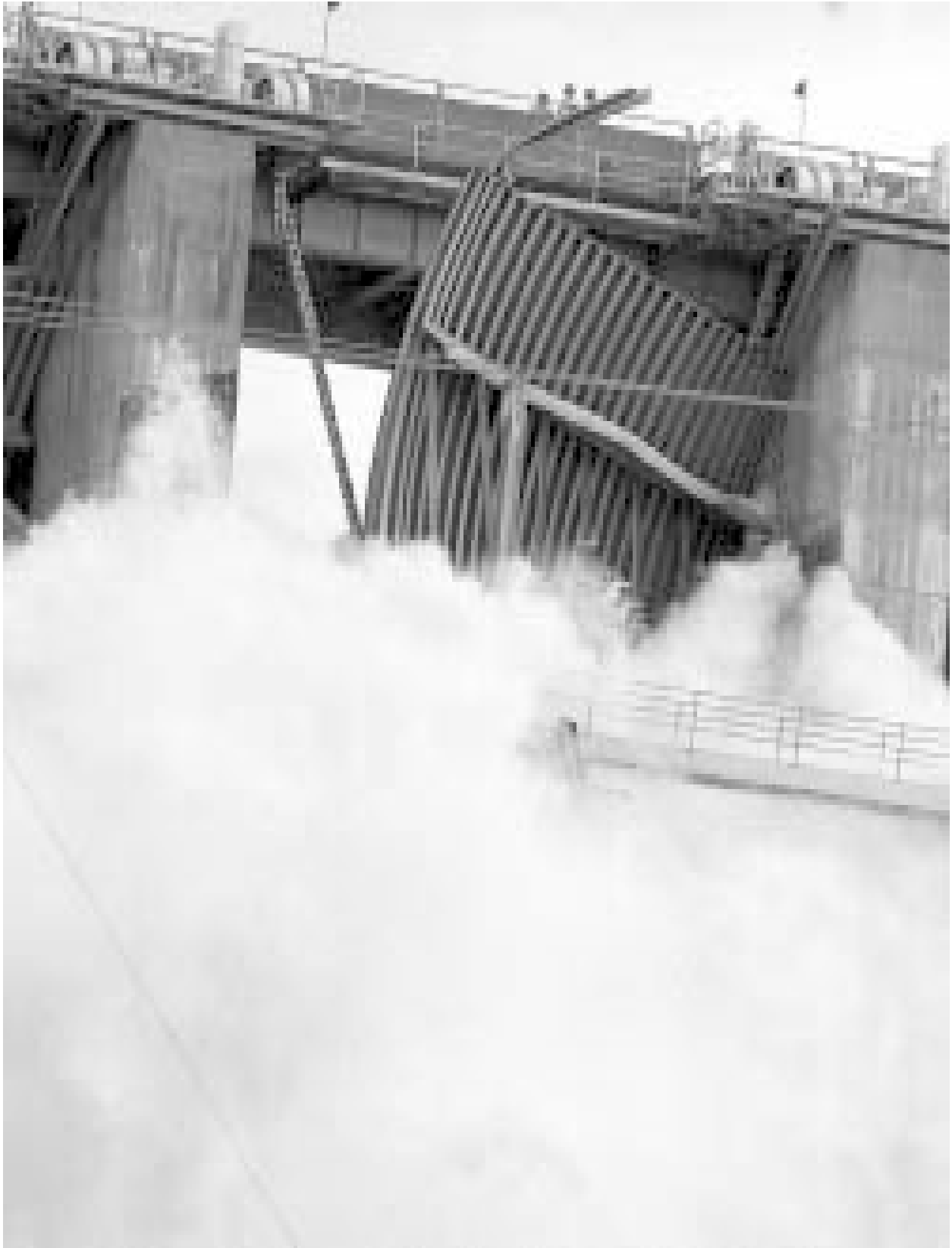
Folsom Dam spillway gate number 3 releasing about 40,000 cubic feet per second on July 17, 1995. The gate is open at 45 degree angle.
