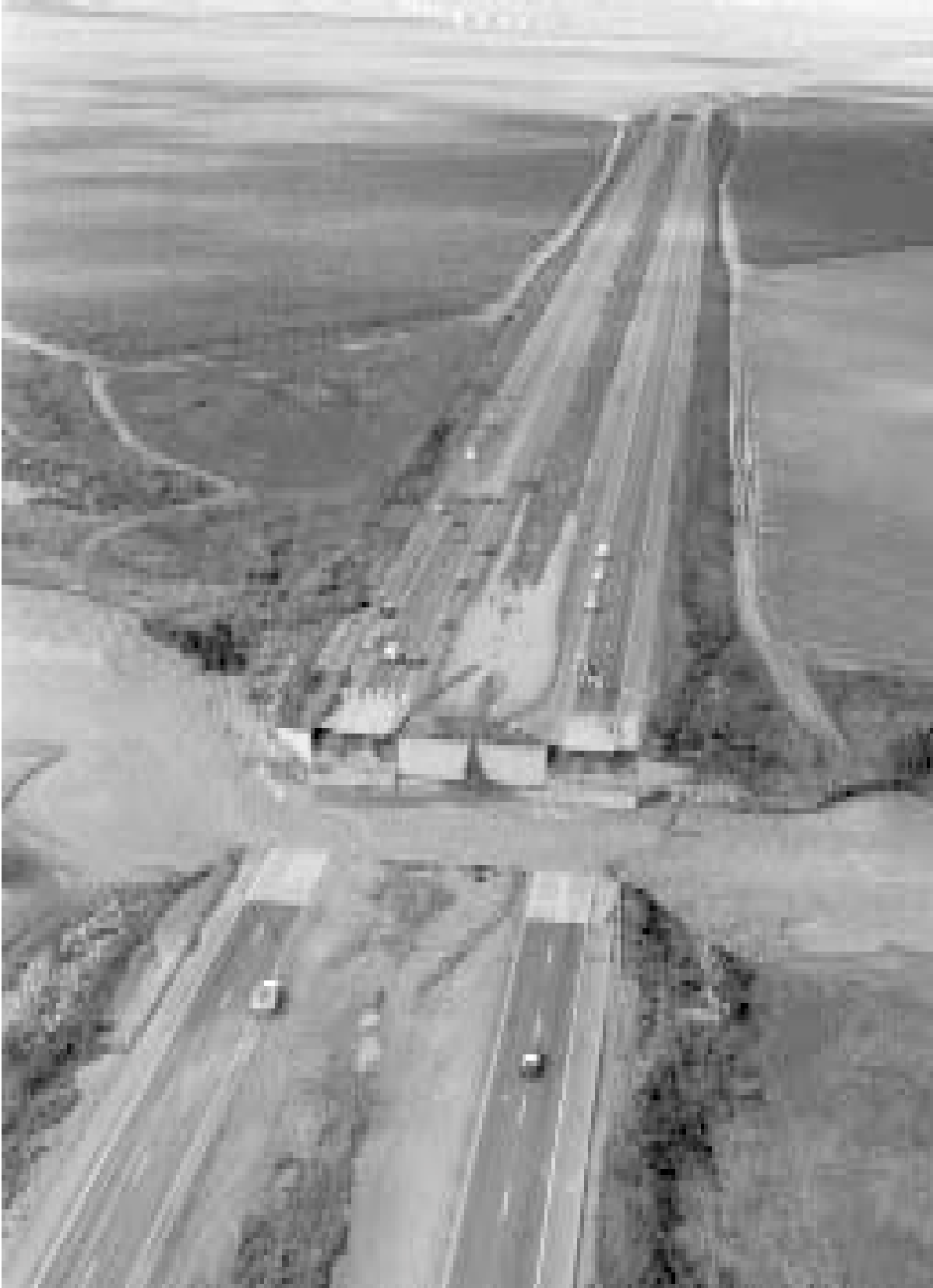
Floodwaters from the Arroyo Pasajero washed out a 100-foot section of Interstate 5 near Coalinga on March 10, 1995. (AP/Wide World Photos)
