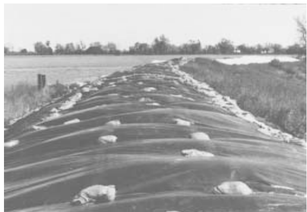
Cache Creek North Levee on March 29, 1995, approximately a quarter mile below the town of Yolo.
