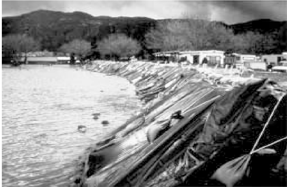
Levee fortification and sandbags placed along Lake Elsinore for the protection of threatened homes.
