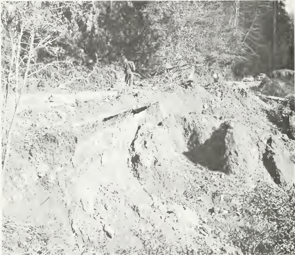
Roadway of State Highway 36 undercut by runoff near the community of Bridgeville, Humboldt County. (DWR Photo)
