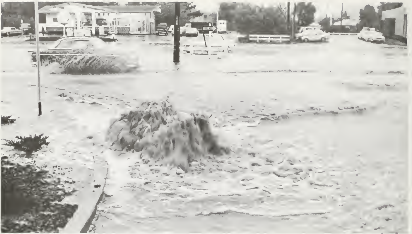
"Popped" manhole in the town of Mill Valley in Marin County on January 18, 1973. (Photo by the San Rafael Independent Journal)
