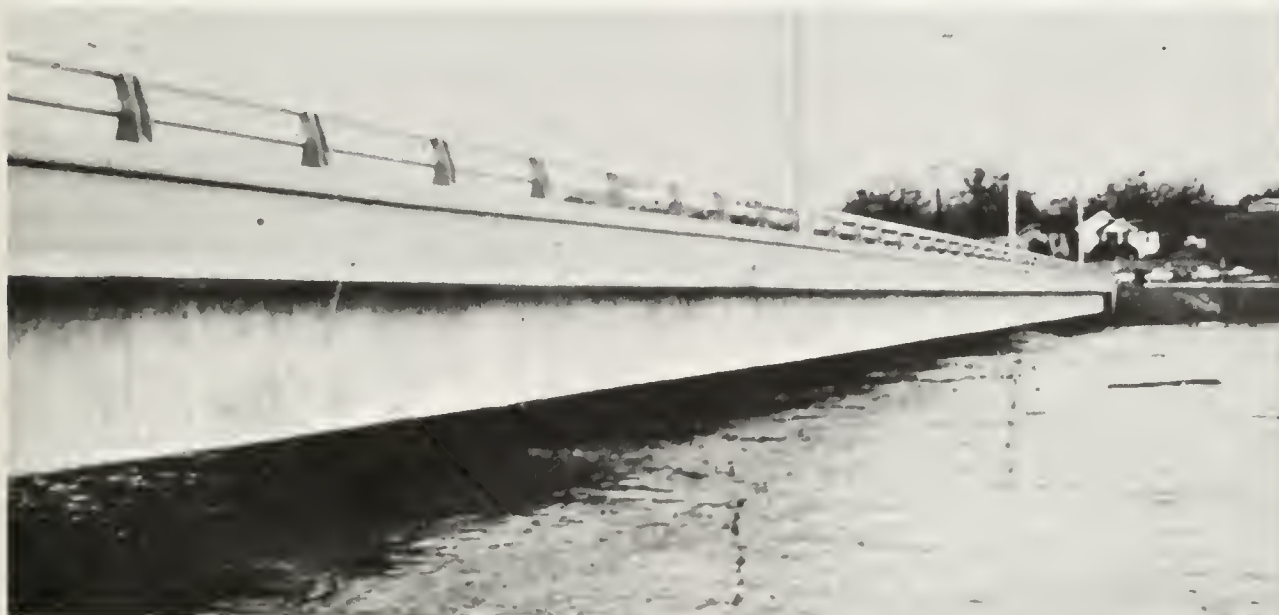
High river flows threatened numerous bridges throughout California. Photograph - courtesy Monterey County Flood Control and Water Conservation District.
