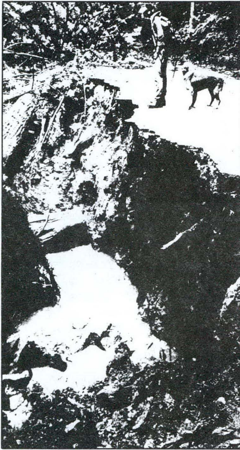
Canyon road washed away
