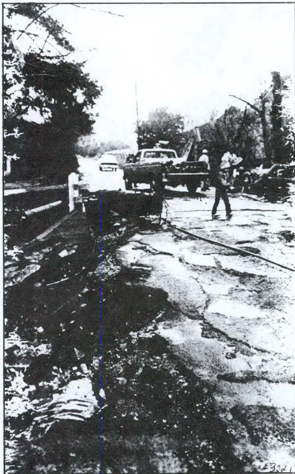
Surface damage to the Glen Canyon Road bridge occurred after a logjam pushed water over the top.
