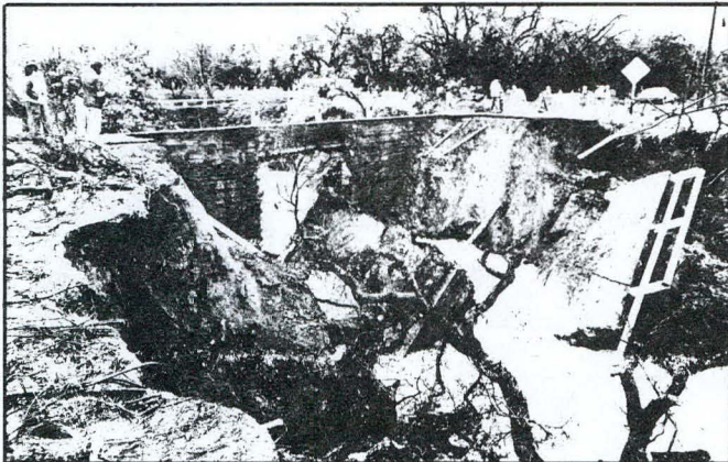
Co. Rd. 79 bridge crumbled into tributary of Cache Creek
