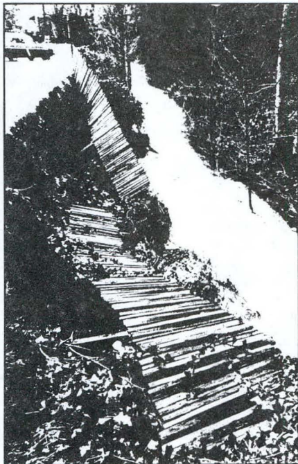
Embankment washed away
