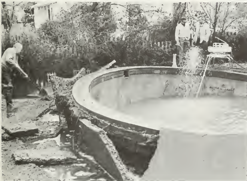
Heavy rains cause problems other than flooding. This swimming pool was floated out of the ground by the rain-soaked soil. Photograph courtesy of The Sacramento Bee.
