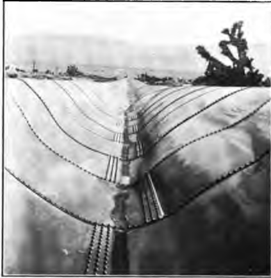
Collapsed Antelope Siphon
