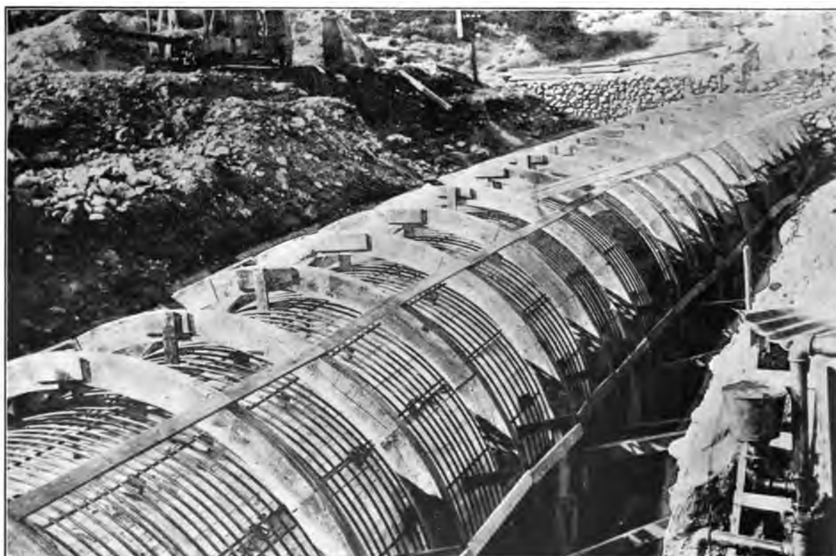
Concrete Siphon in Whitney Canyon. Photograph shows wooden forms. These were supplanted on other concrete siphons by steel forms
