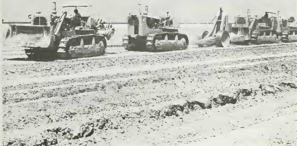
Ripping hardpan soils to a depth of 5 to 7 feet Collin Company photo
