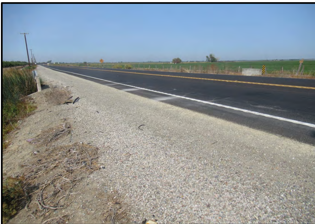
Potential GDE #18124, looking northwest at Maze Boulevard; 09/15/21. This potential GDE is primarily comprised of the road and road shoulder, and also includes a portion of an agricultural drain and part of a leveled field.
