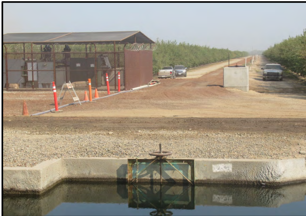
Outlet from the MID lateral and adjacent groundwater well that provide water to Riley Slough via a pipeline, looking north; 09/15/21.
