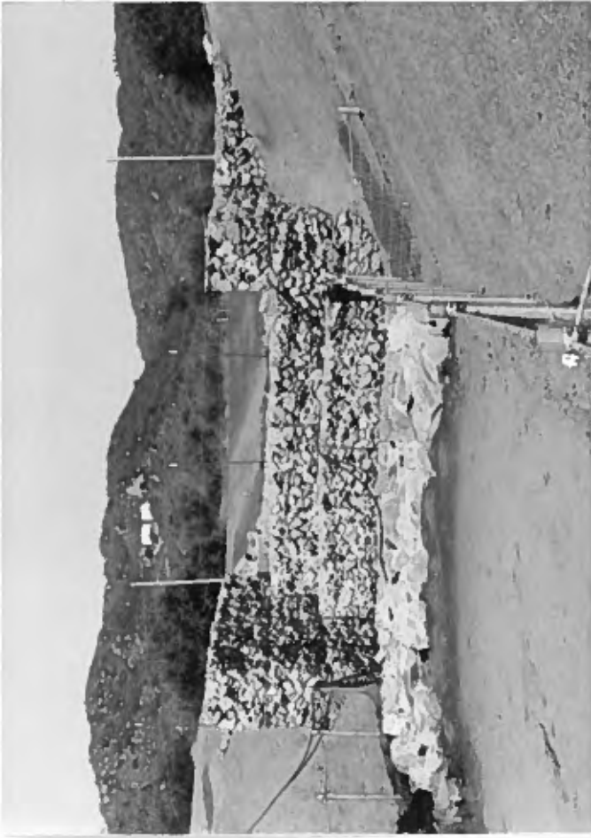
USLRRCD and NRCS constructed dam and culvert on Rincon Reservation in order to prevent flooding of Paradise Creek Road
