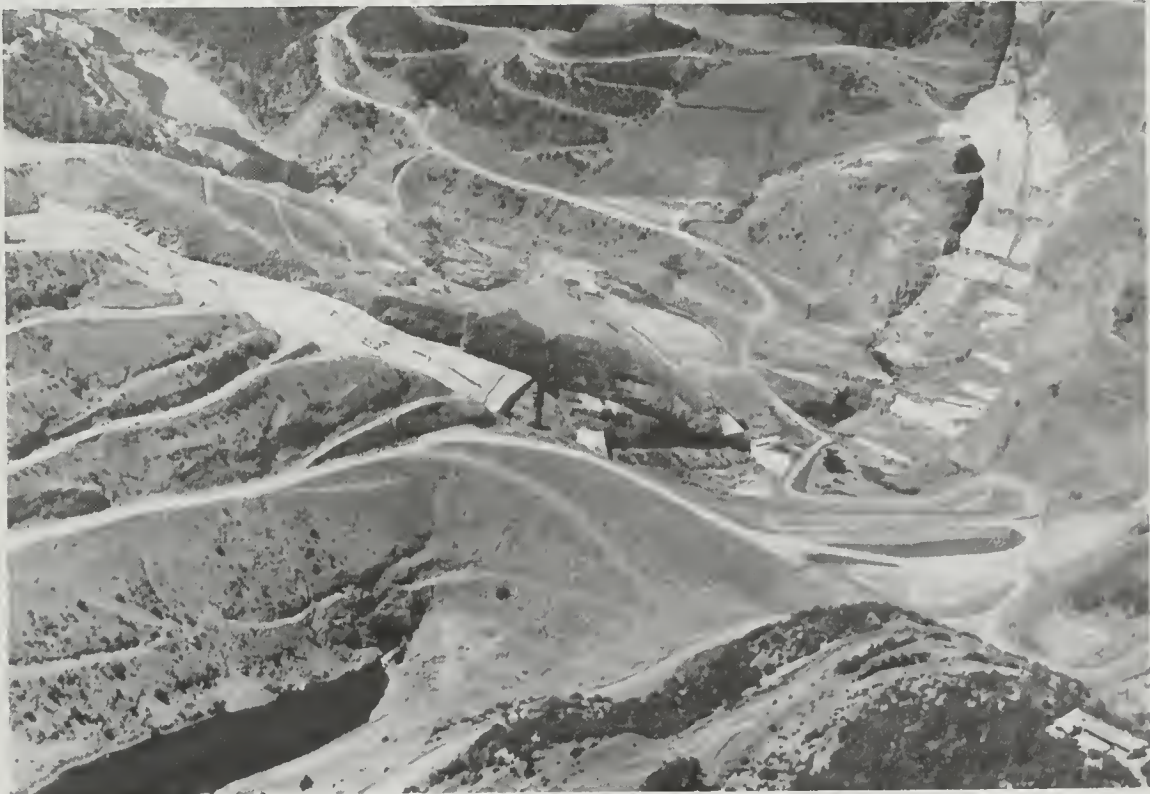
Auburn Dam site on the North Fork American River. Downstream view shows the present status of construction. A 200-foot-high upstream cofferdam is situated in the foreground, with the dam's keyway or "notch" in the canyon visible just above. Work on the dam has been suspended, pending redesign to meet higher seismic criteria and reauthorization by Congress.
