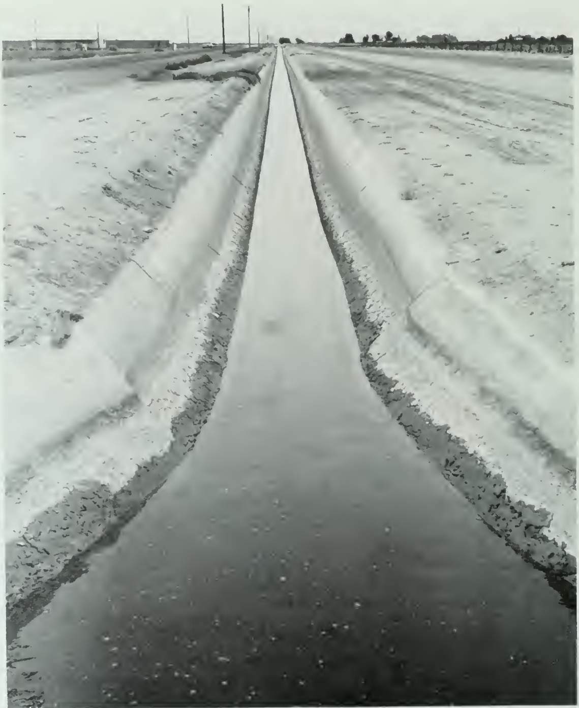
Lining ditches and canals is a major element in the continuing effort by the Imperial Irrigation District to reduce waste of water.
