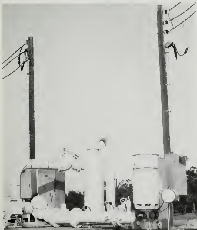
Today most ground water is extracted by deep well turbine pumps from depths of 100 feet or more.
