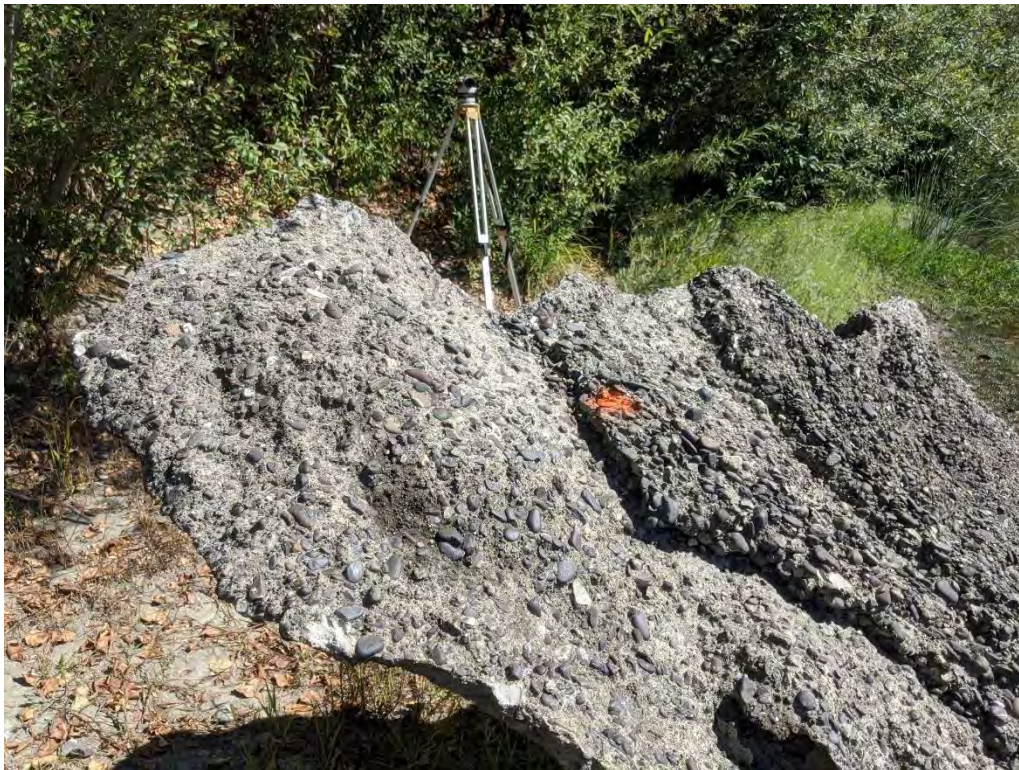
Figure 5. BM2 at R-5: blaze spot on concrete rip-rap
