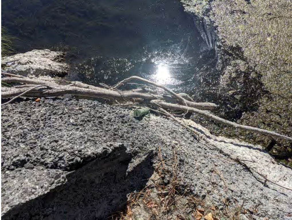
Figure 4. BM1 at R-5: upstream (left) anchor bolt
