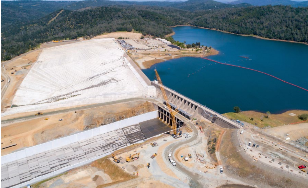
Figure 3. Aerial View of Reconstructed FCO Spillway Chute and Roller-Compacted Concrete Apron on Emergency Spillway (DWR 2019)
