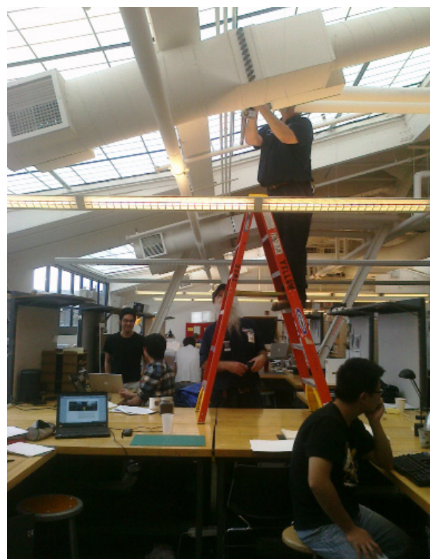
Figure 7.4: ASHRAE’s Standard 180 for quality maintenance of HVAC systems is a good example of a professional standard of care. It provides a lengthy checklist of items a mechanic must check and ensures accountability for carrying out the process. (Photo: Aaron Plewke, flickr , licensed under Creative Commons license 2.0)
