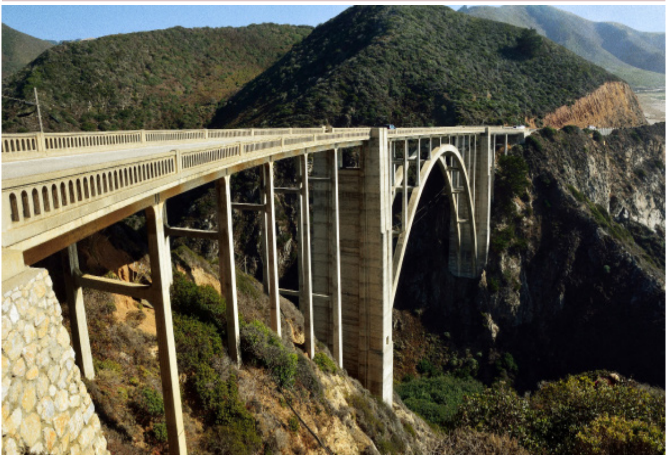
Figure 1.3 Developing climate-safe infrastructure requires the establishment of a strong bridge between science and the engineering community, as well as supportive public policy aligned with the goals of resiliency. (Photo: Bixby Bridge near Big Sur, CA; Russell Mondy, flickr , licensed under Creative Commons license 2.0)
