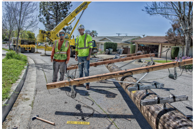
Figure 9.2: Workforce development must reach into all segments of California society, and particularly open doors to minority, women and otherwise previously disadvantaged workers. (Photo: Workers erecting a telephone pole; Russ Allison Loar, flickr, licensed under Creative Commons license 2.0)
