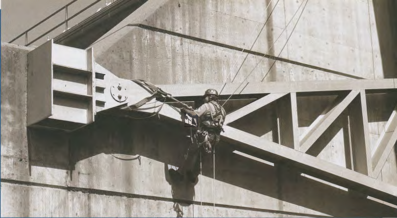
A Division of Safety employee checks a radial gate on Thermalito Diversion Dam.
