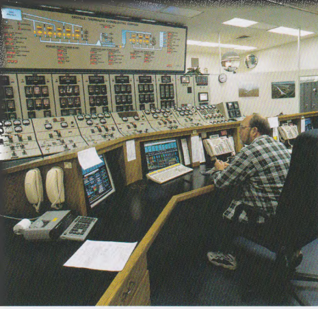
Field division Area Control Center.
