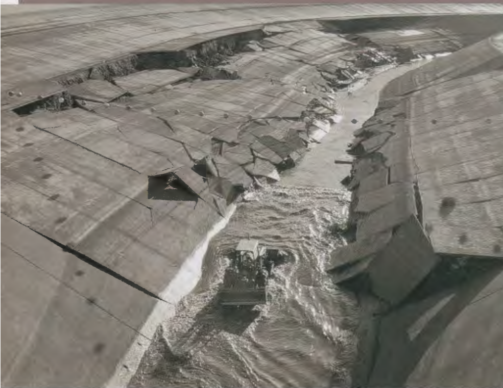
Canal lining failure along the East Branch Aqueduct.
