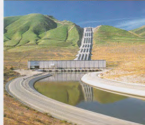
Chrisman Pumping Plant
