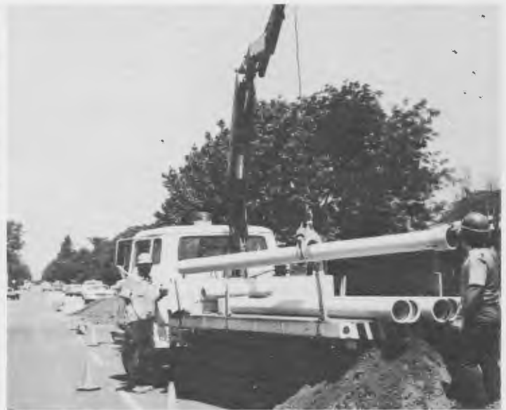
Mesa Consolidated crew takes new pipeline from truck. System maintenance aids customer relations.
