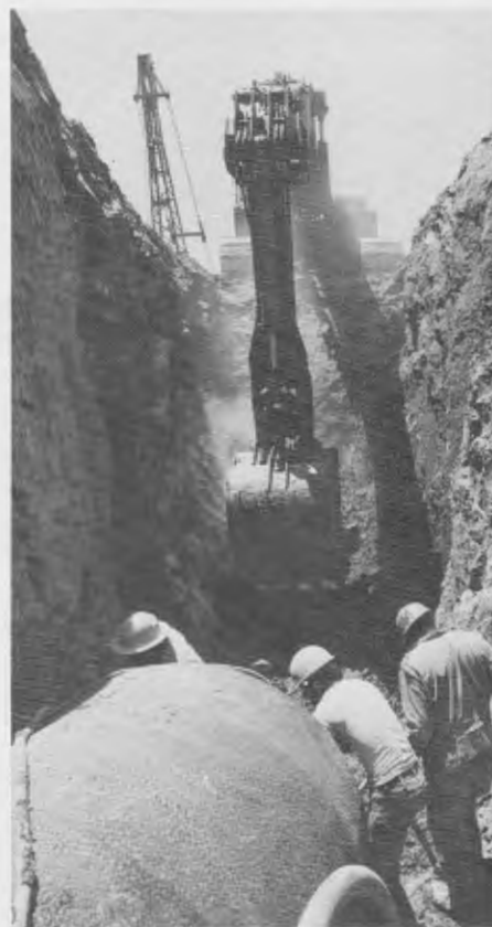
Trencher above opens the way for East Bay's Moraga Aqueduct during project's construction.
