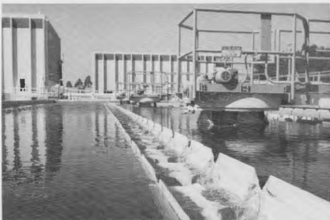
Orange County water District's Water Factory 21 recycles water previously dumped into the ocean.
