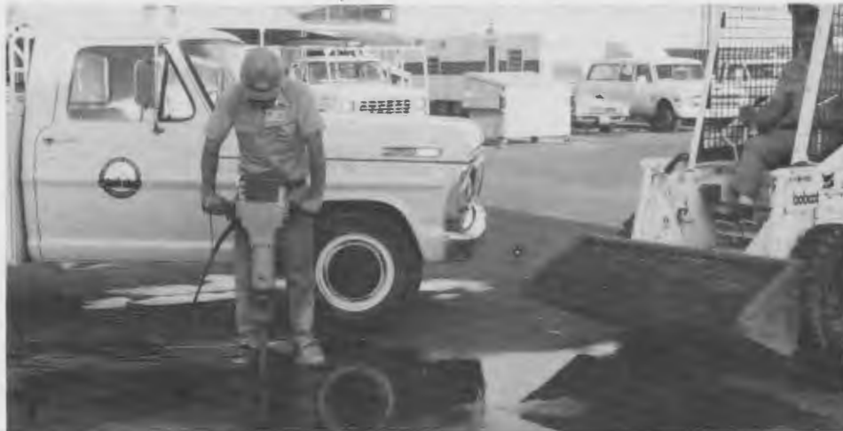
Work proceeds on line leak in Arcade County Water District system. Quick response for such repairs help maintain customer satisfaction.
