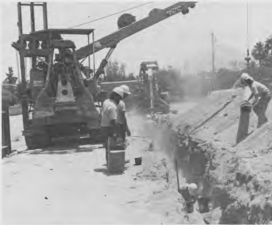
Coachella Valley County Water District crew installs an urban water line in Palm Desert, part of the district's system upgrading program.
