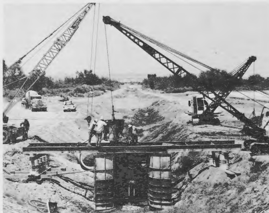
Crew of Imperial Irrigation District proceeds with installation along the district's distribution canal in agricultural rich Imperial Valley.
