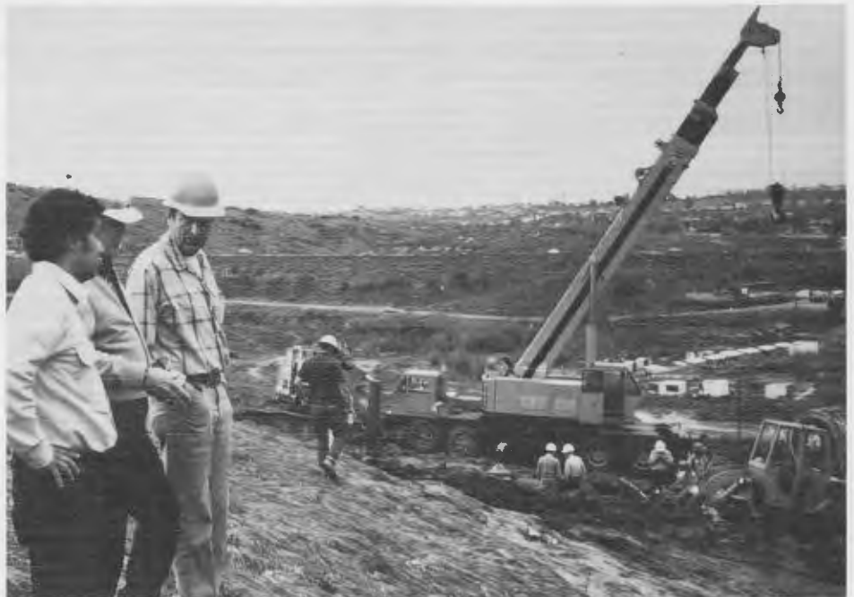
Crews from San Diego County Water Authority and Otay Municipal Water District repair pipeline failure near Sweetwater Reservoir.
