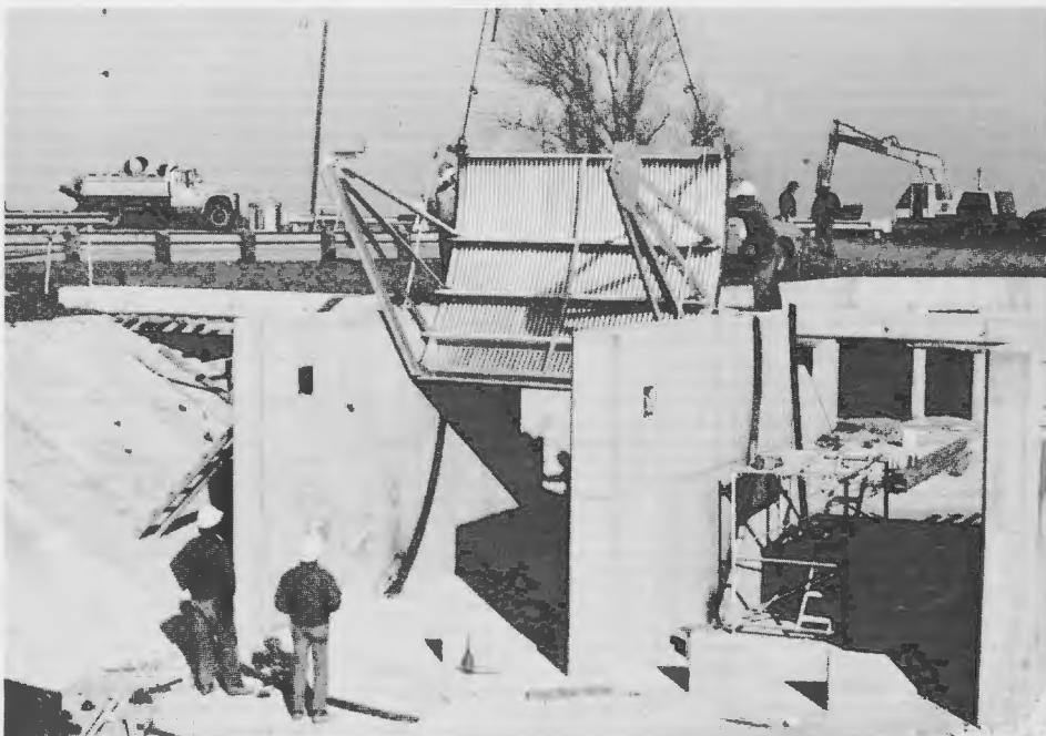
Glenn-Colusa Irrigation District crew installs radial gates to complete enlargement and modernization of check and siphon structure.
