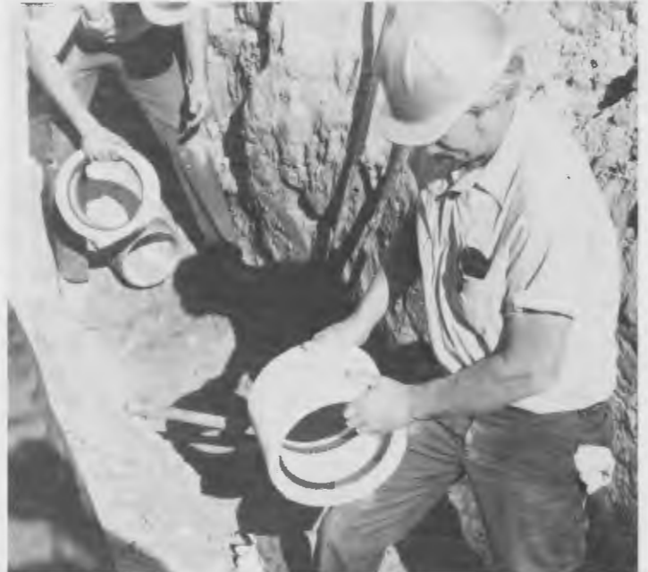
Yorba Linda crewmen install a new line as part of activity to repair major water line.
