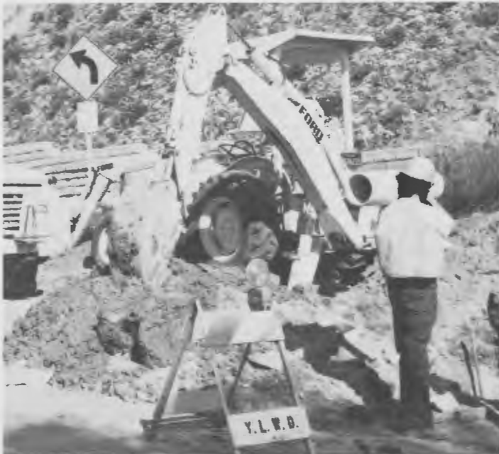
Yorba Linda County Water District crew prepares trench for repair of a major water line.
