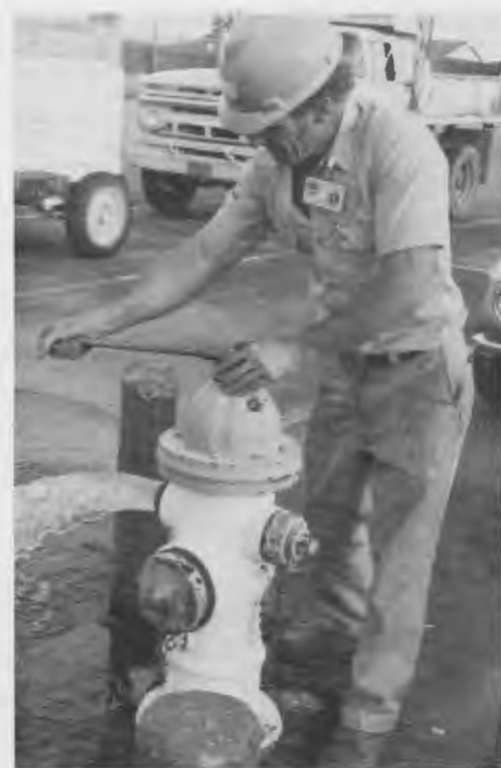
Arcade crewman inspects flow at local fire hydrant.
