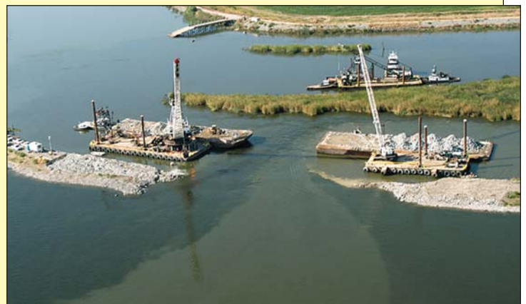
In June 2004, a levee along Jones Tract (ten miles west of Sacramento) failed without warning, flooding almost 12,000 acres of farmland and illustrating the continued long-term risk of the existing Delta levee system. Its failure forced a brief change in normal Delta water project operations, and provoked increased water quality and fisheries monitoring. Soon after the breach occurred, U.S. Geological Survey scientists measured a maximum tidal discharge of 19,000 cfs at the opening. By the time workers had almost completed closing the breach, maximum tidal flows had decreased to about 10,000 cfs. Data from the long-term flow station located on Middle River showed substantial increases in the tidal velocities after the failure, a potential threat to other weak spots. More in-depth analysis of the impacts will be shared at a special session of the CALFED Science Conference in October 2004. Source: DWR
