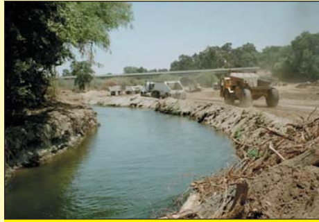
To ease excavation, the restoration design called for the creation of a temporary river bypass channel, so the equipment could more easily fill in the pool and recreate the old channel.
