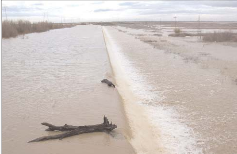
Raising the height of this outlet weir is one of a number of possible improvements to a 1930s-era settling basin where Cache Creek empties into the Yolo Bypass near the city of Woodland. The basin traps an estimated half of the mercury coming downstream in wet years.
