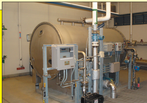
Ozone generator at the Contra Costa Water District's Bollman Water Treatment Plant near Concord. Source: CCWD
