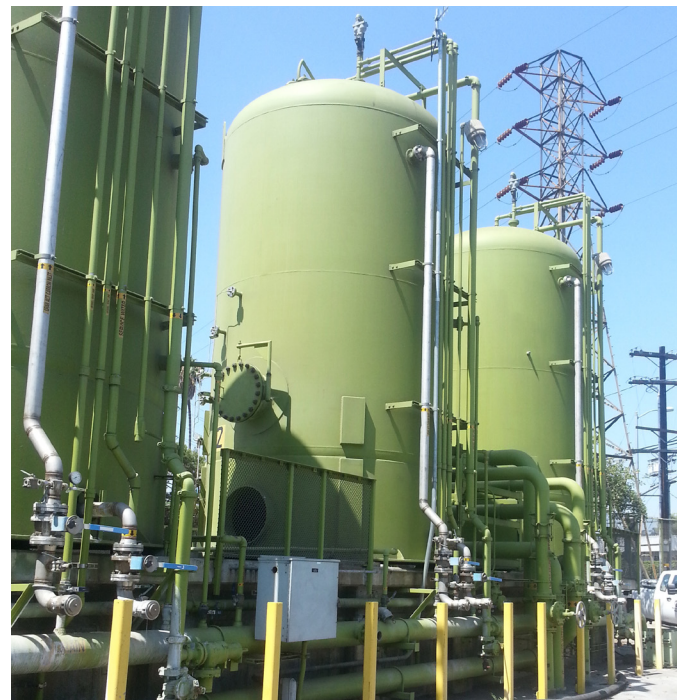
LADWP granular activated carbon treatment at Pollock Well Field (1999)
