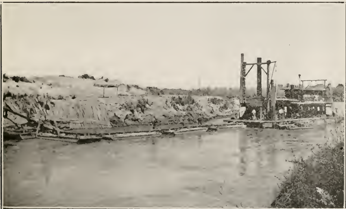
FIG. 2. Dredging silt from Imperial Canal; a major item of irrigation maintenance in Imperial Valley.
