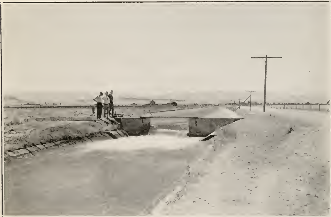
FIG. 2. A concrete-lined irrigation canal on the Orland Project of the United States Reclamation Bureau.
