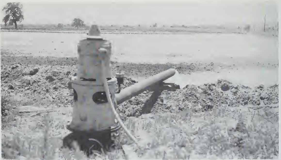
Ground Water Pumping Well in San Joaquin Area
