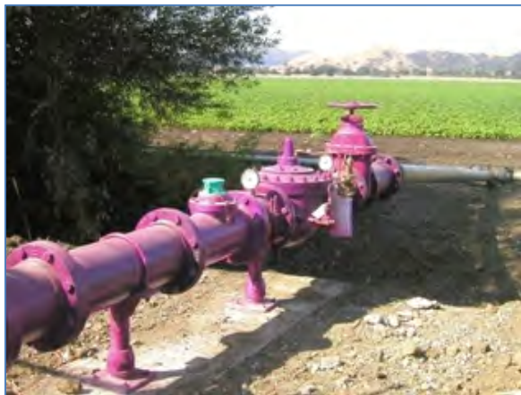
This pipeline in Gilroy provides recycled water to a local farmer
