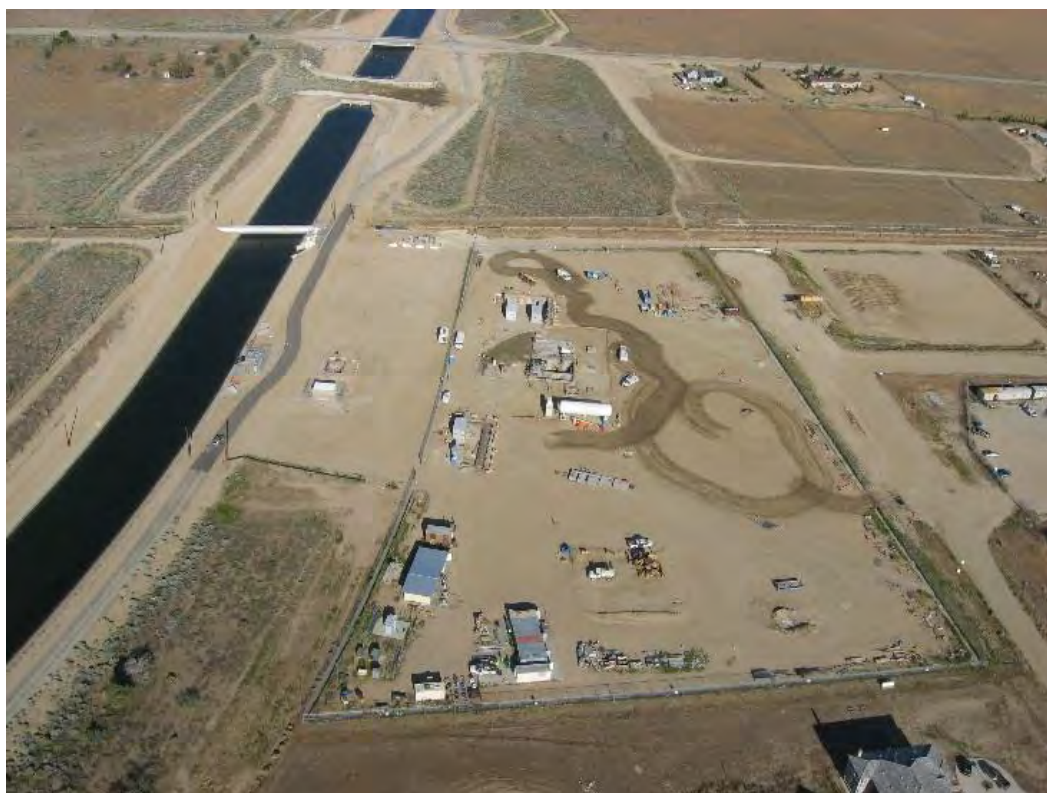
Neenach Temporary Pumping Station, construction site, looking northerly, taken May 4, 2015, by Aqueduct Aerial Patrol.
