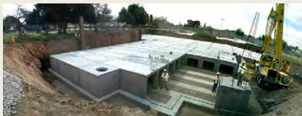
Underground infiltration gallery in Garvanza Park
