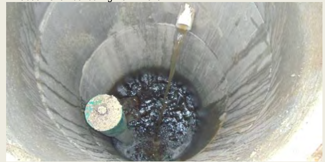
Infiltration Chamber during Rain Event
