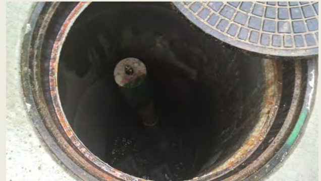
Infiltration Chamber during Rain Event
