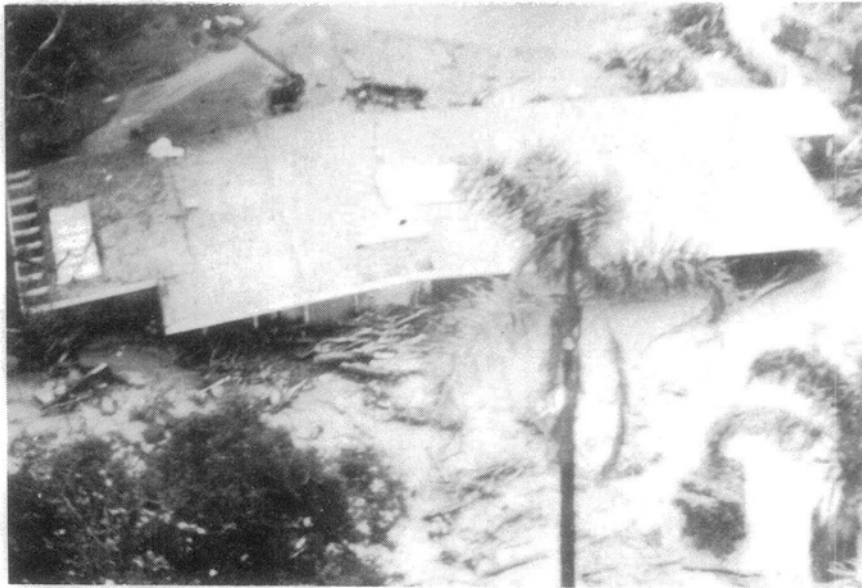
Figure 18 — Overflow from San Ysidro Creek, in the Glen Oaks area, during January 1969 flood.
