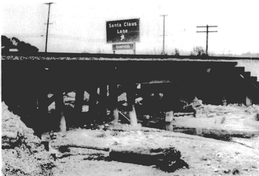
Figure 7 — Southern Pacific Railroad bridge over Arroyo Paredon (looking upstream at river mile 0.10).
