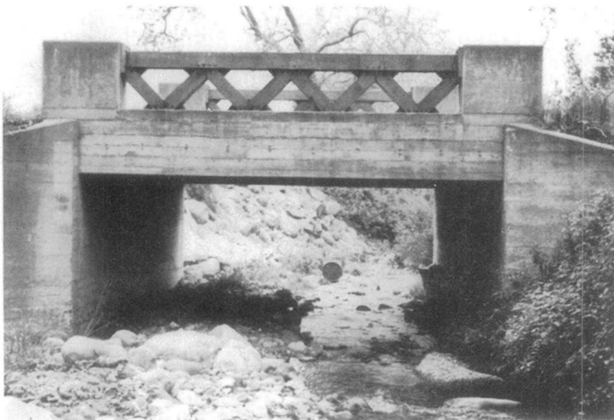
Figure 3 — Sheffield Drive bridge over Romero Canyon Creek (looking downstream at river mile 0.74).
