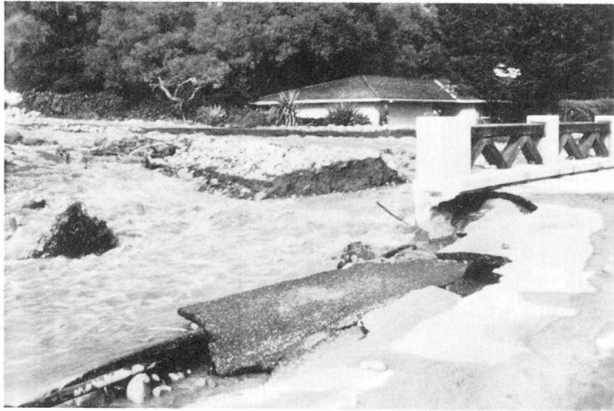
Figure 16 -- San Ysidro Creek, at East Valley Road, during January 1969 flood. The channel was filled with rocks and debris forcing flow out of the banks.
