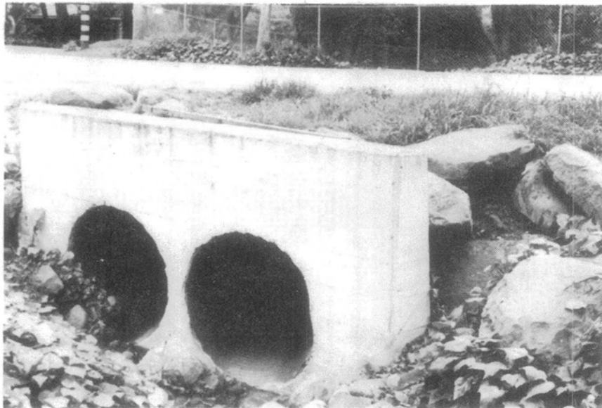
Figure 4 — East Branch Buena Vista Creek culvert at Veloz Drive (looking downstream at river mile 1.33).
