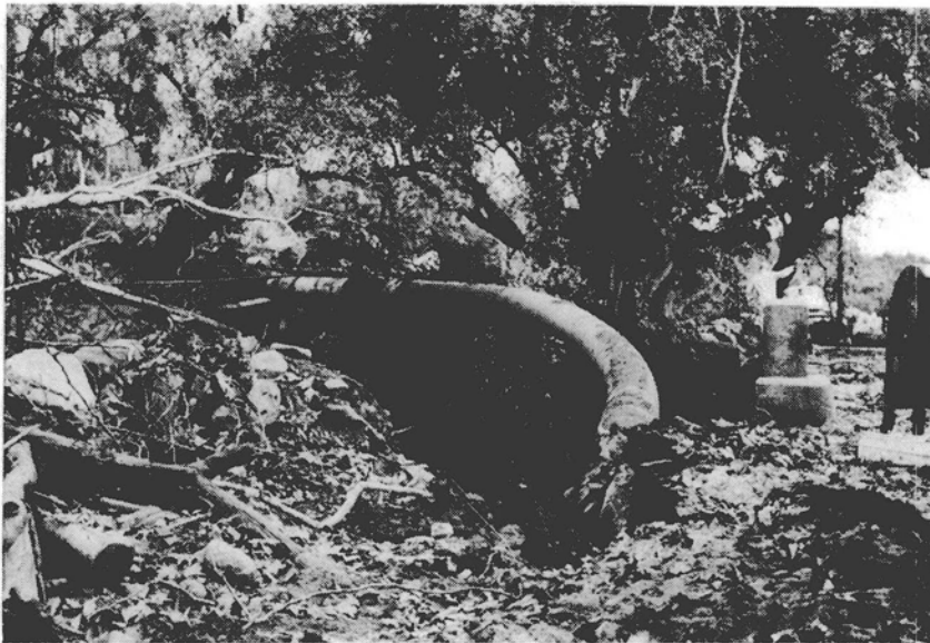
Figure 12 — San Ysidro Creek, near Mountain Drive, after November 1964 flood where a 20-inch high pressure gasline was bent by the force of the flow. Debris were carried over the bridge deck shown on the extreme right of the picture.
