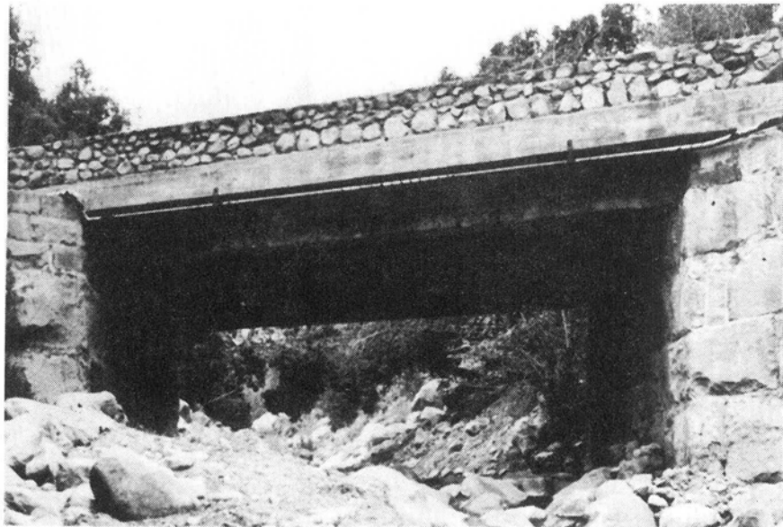
Figure 6 — East Valley Road bridge over West Branch Toro Canyon Creek (looking upstream at river mile 1.85).
