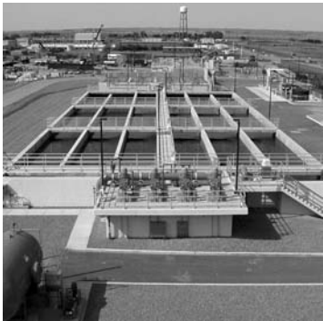
The 12.8 mgd Recycled Water Facility of Delta Diablo Sanitation District treats recycled water for landscape irrigation and for cooling towers at electrical power stations in Pittsburg, CA.
