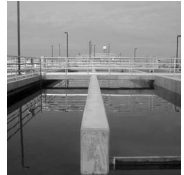
Chlorination contact basin at Delta Diablo Sanitation District Recycled Water Facility in Antioch, CA, ensures a recycled water that is essentially free of pathogens.
