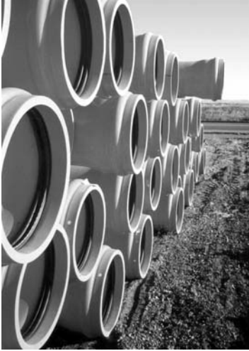
Purple colored pipes ready for installation to deliver recycled water. Purple has been designated for the piping used for recycled water in the California Health and Safety Code Section 116815.
