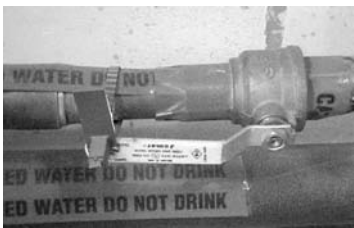
To help ensure against cross-connection between potable and recycled water lines in buildings, purple tape covers recycled water pipes and breakable seals are placed on valve handles to detect when water was shut off to perform plumbing changes. A log book is required to record all seal breaks and the plumbing work performed.
