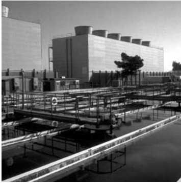
Water Factory 21, operated by Orange County Water District, provides up to 15 mgd of tertiary and advanced treatment of recycled water injected into an aquifer for groundwater recharge and a seawater intrusion barrier. This has operated since 1975.
