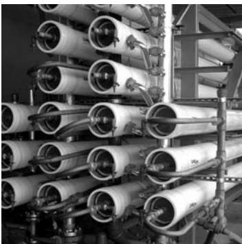
Reverse osmosis is an advanced treatment technology that is used in certain situations where a high degree of pathogens or chemicals must be removed, especially in indirect potable reuse and industrial applications.
