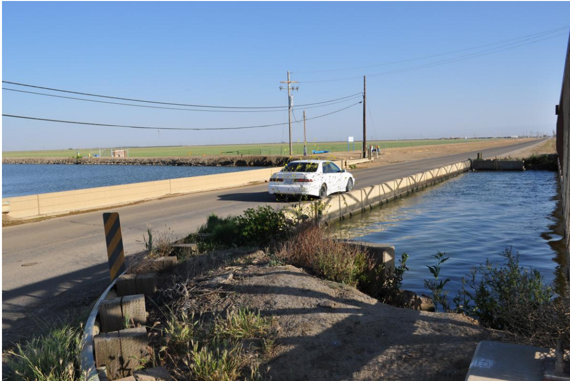
Figure 6. The partly submerged Russell Avenue bridge over the Outside Canal north of Mendota, California. Before subsidence, canal inspections by Central California Irrigation District staff were conducted from a boat passing under the bridge.
