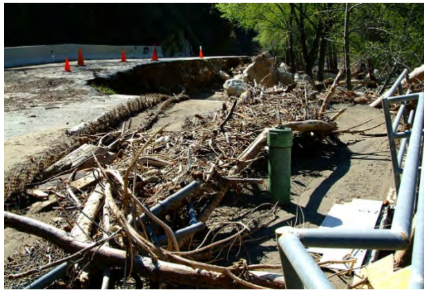
Figure 41: Road damage after flooding, wildfire or landslides are just some of the risks from climate change to transportation infrastructure.
