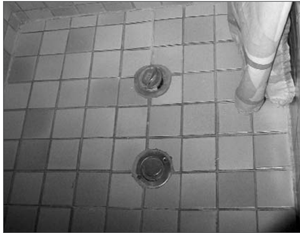
Water inside, reused outside: Dual drains installed in a second-story shower allow water to be diverted to the garden.
