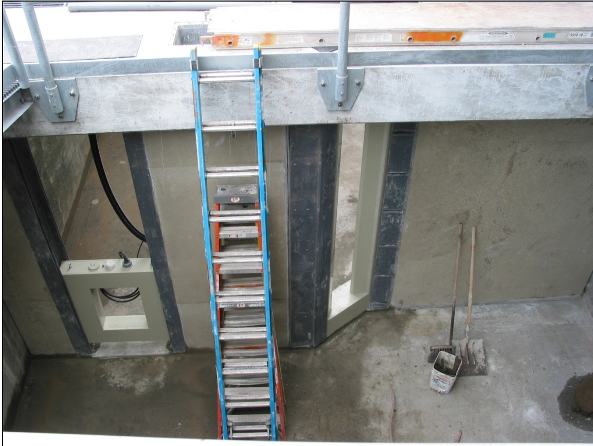
Figure 134: Lower Granite Dam Fish Ladder: Vertical slot and weir orifice antennas during installation (Courtesy of PTAGIS)
