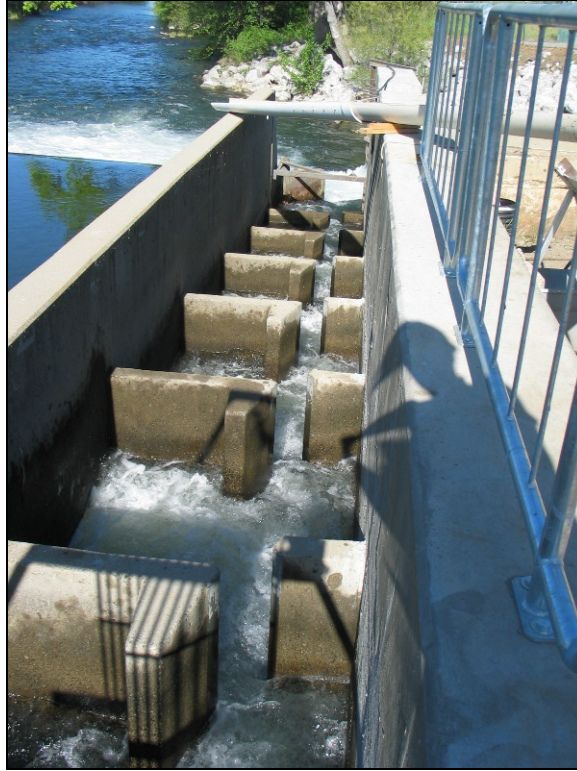
Figure 17: Vertical Slot Fishway at Coleman National Fish Hatchery (CA Department of Water Resources)
