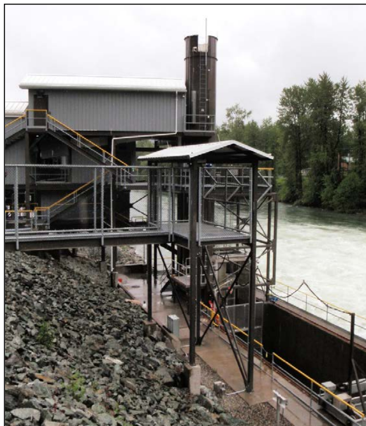
Figure 65: Holding pond #2, brail pond, and fish lock (CA Dept. of Water Resources)
