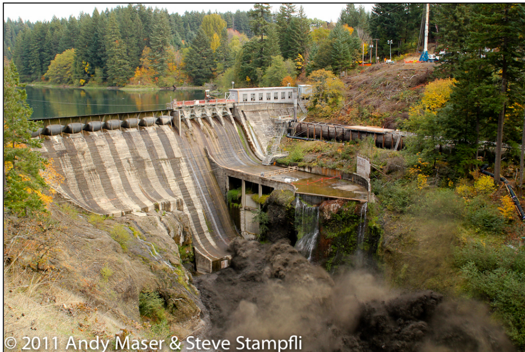
Figure 234: The Breaching of Condit Dam (Courtesy of Andy Maser and Steve Stampfli)
