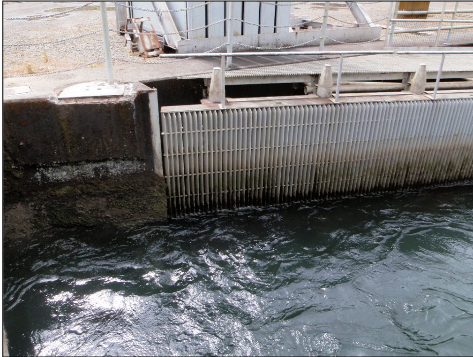
Figure 97: Mayfield Downstream Migrant Collection Facility Louvers (CA Dept. of Water Resources)
