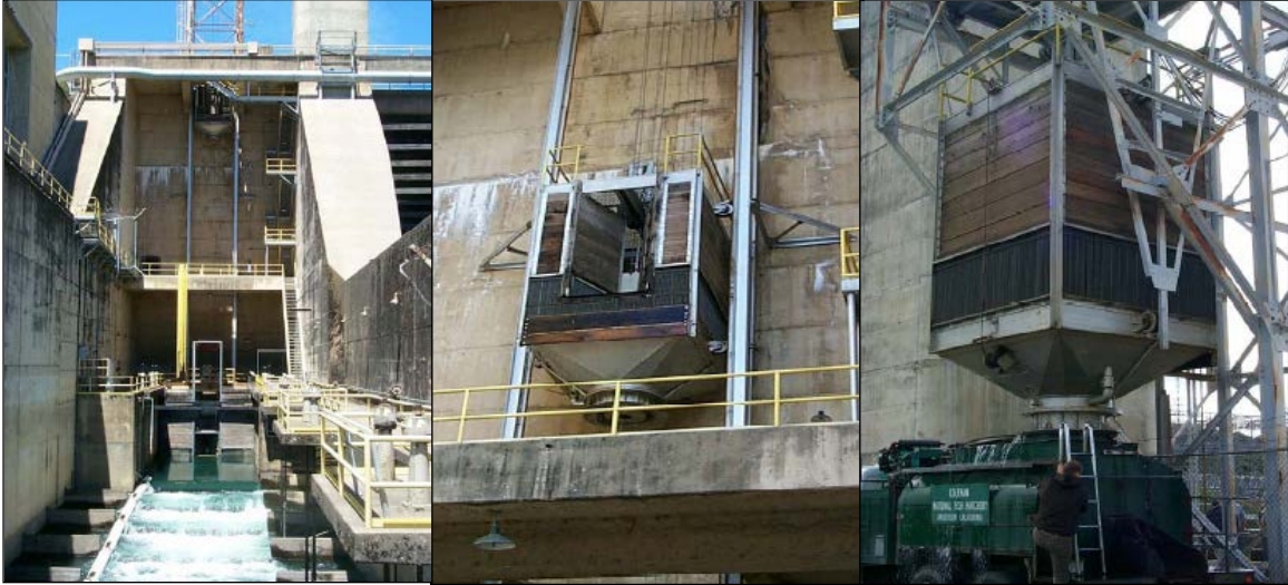
Figure 30: Collection and transport facility at Keswick Dam in California
