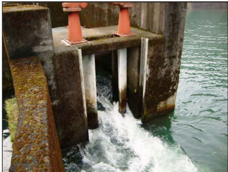
Figure 167: North Fork Fishway Entrance (PGE 2012b)
