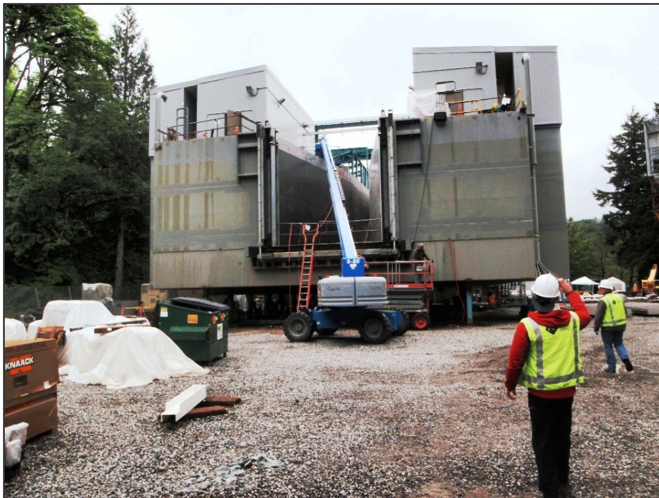
Figure 77: New FSC for Lake Shannon - Upstream side showing primary fish screens (CA Dept. of Water Resources)
