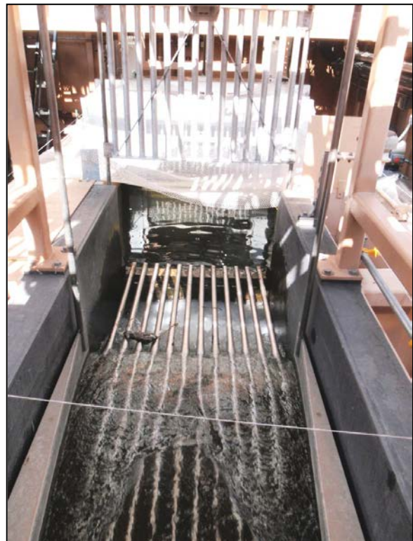
Figure 194: Large Fish Separator (CA Dept. of Water Resources)
