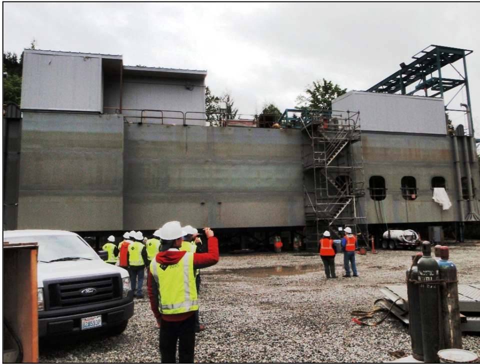
Figure 78: New FSC for Lake Shannon – Side view showing water exit ports (CA Dept. of Water Resources)
