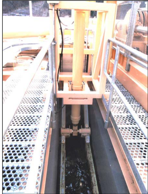
Figure 193: Secondary Fish Screen Channel and Cleaning System (CA Dept. of Water Resources)
