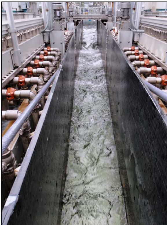
Figure 75: Upper Baker Dam FSC secondary fish screens - looking upstream (CA Dept. of Water Resources)
