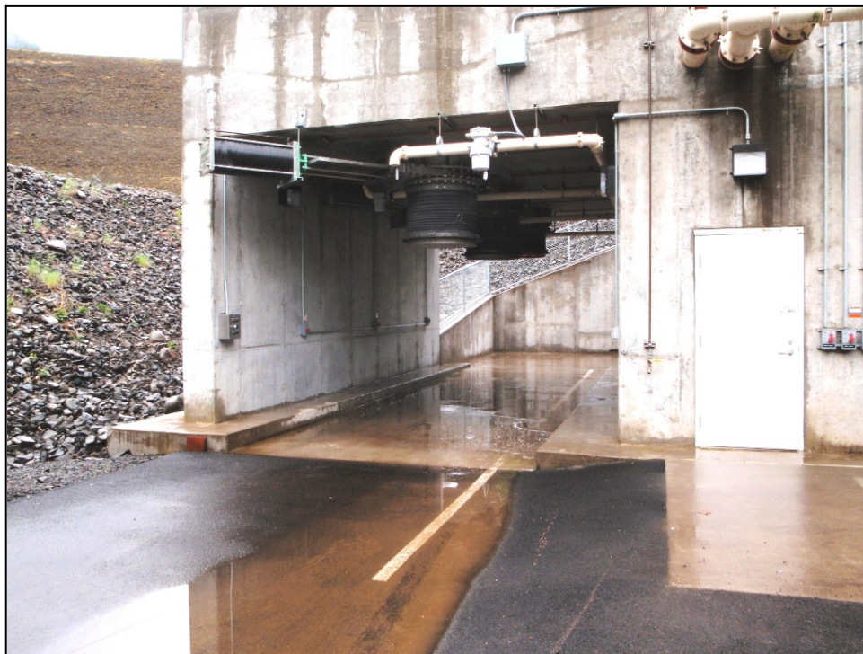
Figure 155: Truck Loading Area (CA Dept. of Water Resources)
