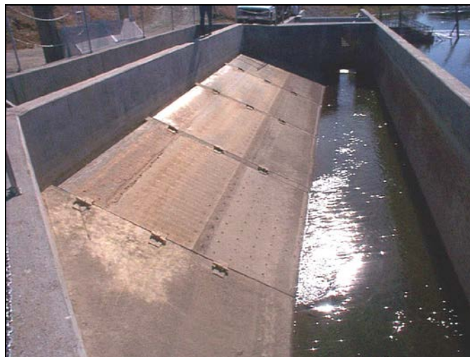
Figure 46: Rancho Esquon Inclined Flat-plate Fish Screen, Butte Creek, CA – Shown at a low forebay elevation (CA Dept. of Water Resources)
