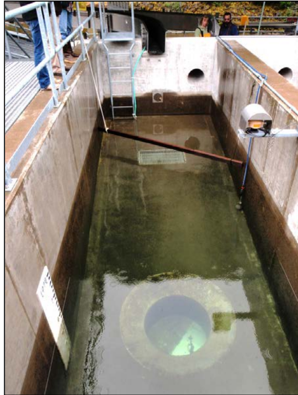
Figure 154: Post-Sort Pool and Fish Loading Port (CA Dept. of Water Resources)
