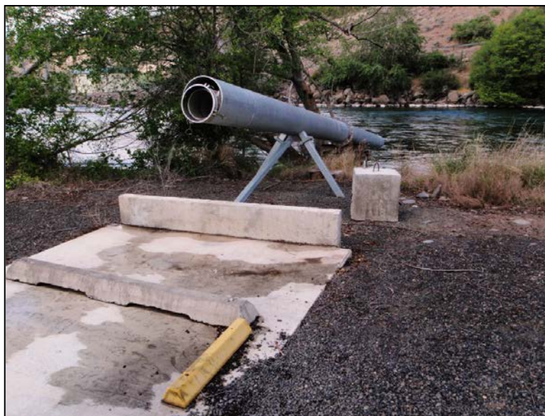
Figure 200: Fish Release Pipe (CA Dept. of Water Resources)
