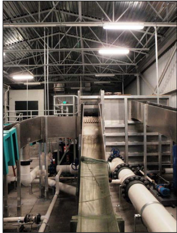
Figure 172: Timber Park Fish Sampling Facility (CA Dept. of Water Resources)
