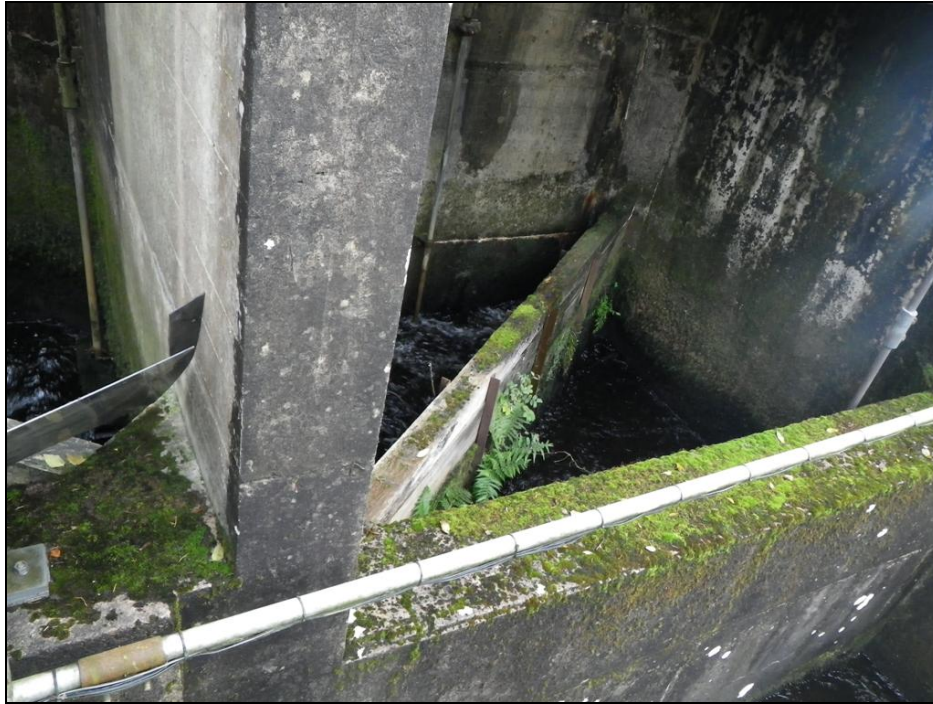
Figure 212. Fish ladder baffle section (within the dam) (Courtesy of Galloway Fisheries Trust)
