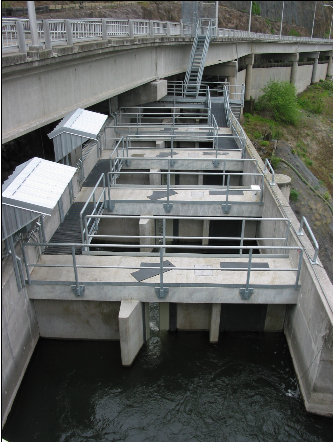
Figure 135: Lower Granite Dam Fish Ladder: Vertical slot and weir orifice antennas after installation, when the ladder is operational (Courtesy of PTAGIS)
