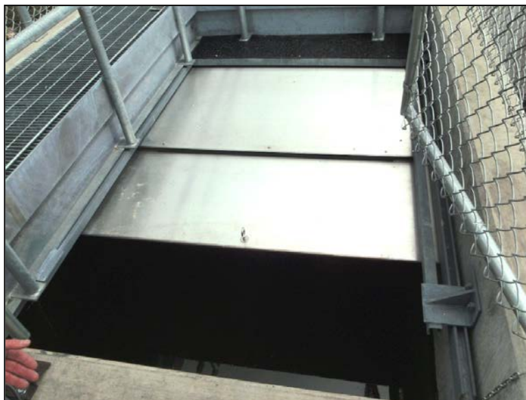
Figure 188: Adult Release Facility (CA Dept. of Water Resources)
