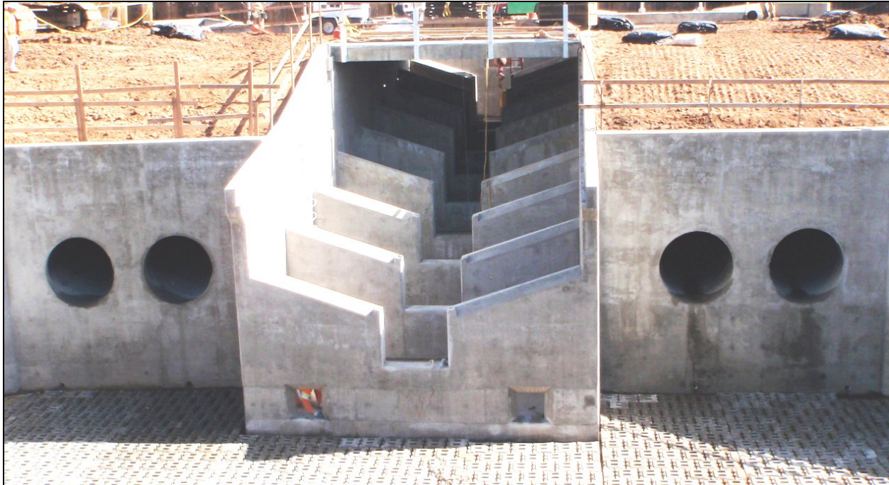
Figure 16: Pool and Chute Fishway at Willow Slough Weir in the Sutter Bypass - Northern California (CA Department of Water Resources)
