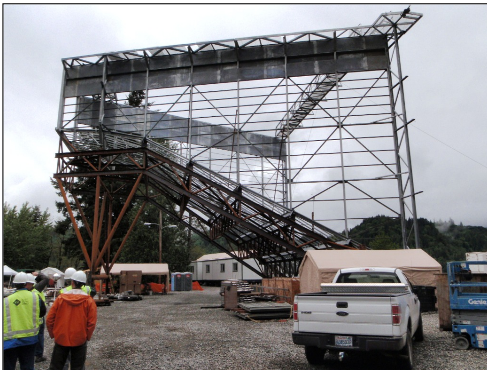
Figure 79: Net transition structure framework for Lake Shannon FSC (CA Dept. of Water Resources)
