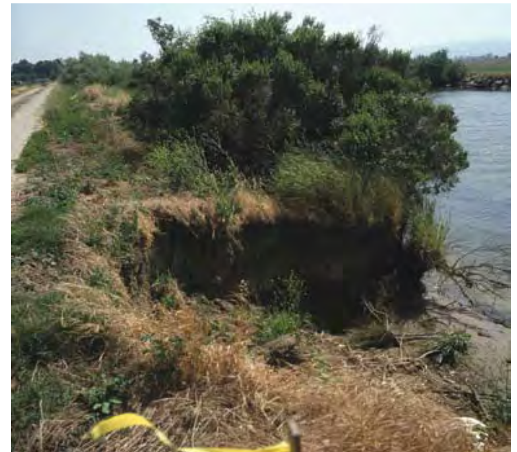
Eroded non-project levee protecting hundreds of acres of agricultural land and wildlife habitat.
