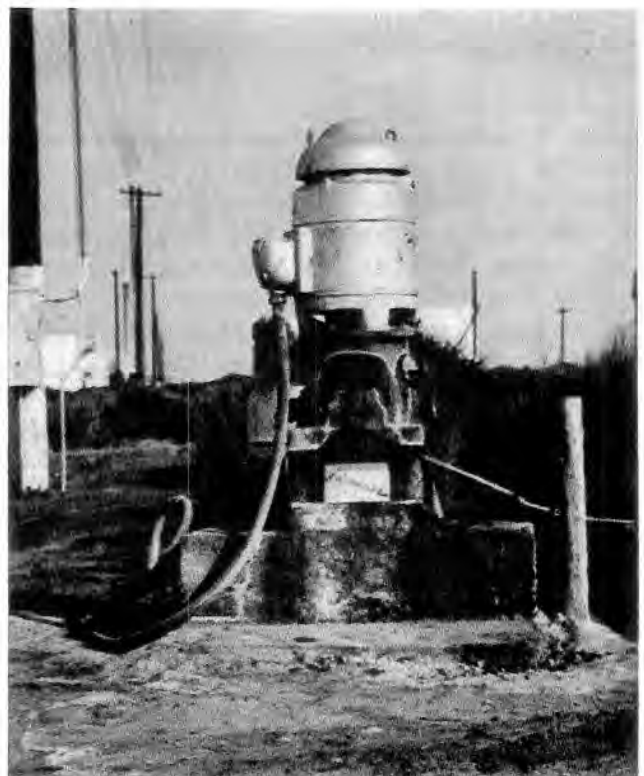
3. Lifesaver for a thirsty land. A typical irrigation pump installation in the San Joaquin Valley. With declining surface storage supplies, more and more farmers turned to ground water to supply their irrigation needs.
