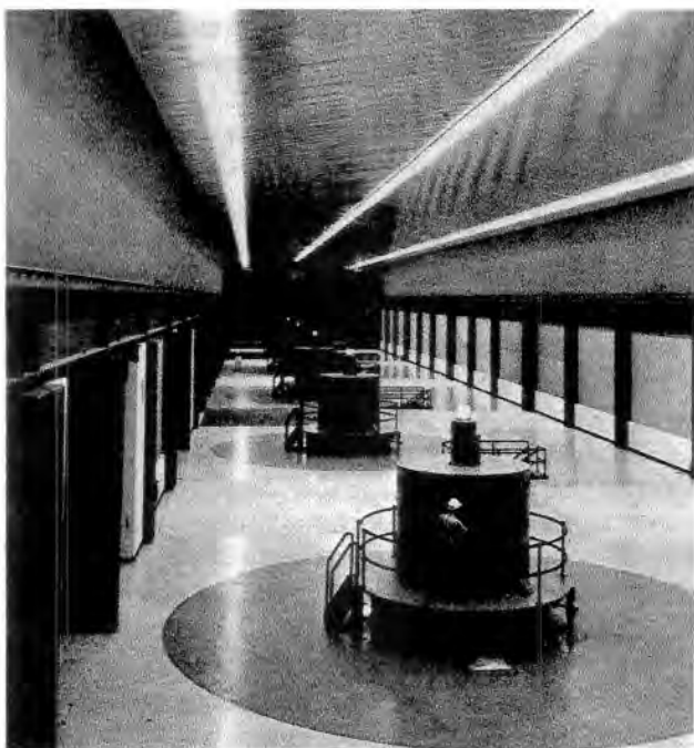
55. Return to normal. Edward Hyatt Powerplant at the base of Oroville Dam, shown here in an interior view, is an example of the hydroelectric generating plants whose power outputs were reduced by drought in 1977 but are expected to produce energy at normal rates in 1978.
