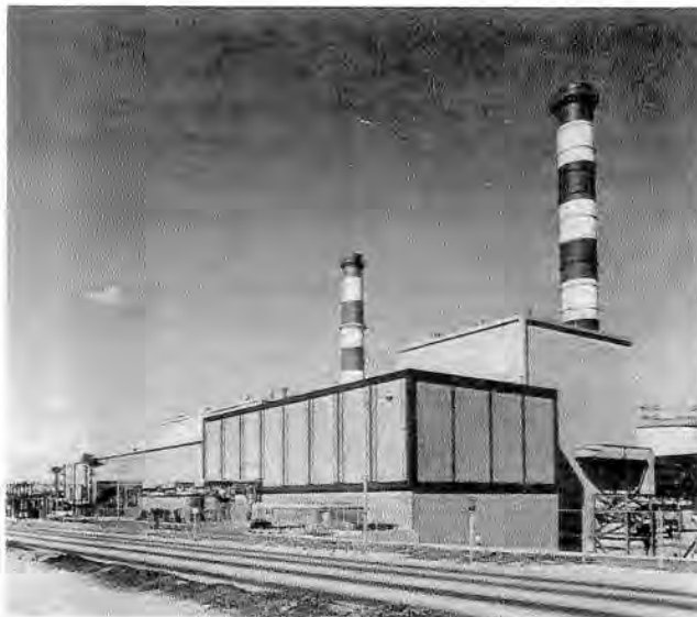
20. Replacement energy. The Scattergood Powerplant, owned and operated by the Los Angeles Department of Water and Power but idled for lack of clean burning fossil fuel, was put into service to meet the critical energy demand in the summer of 1977. (LADWP photo.)
