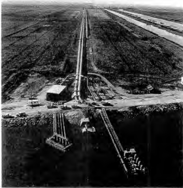
40. An emergency water supply. This aerial view shows the two newly constructed pumping plants in the Sacramento-San Joaquin Delta at Middle River. EBMUD facilities are on the left and DWR's pumping plant appears at the right. Both plants were constructed in 1977 to provide emergency supplies of water pumped from the Delta into EBMUD's Mokelumne Aqueduct, shown stretching west with Mt. Diablo in the distance.
