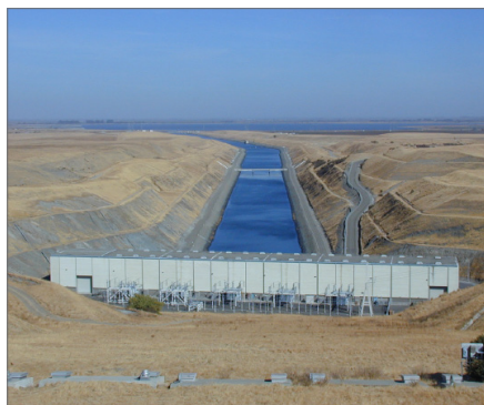
Massive pumping plants in the south Delta draw in water for export. | Both photos Courtesy of Diana Jacobs, SRPT
